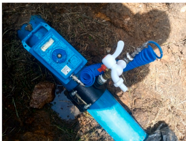
Fig. 2. Sampling point created on the DN100 pipeline with a pressure logger installed and tap point to collect water sample.
