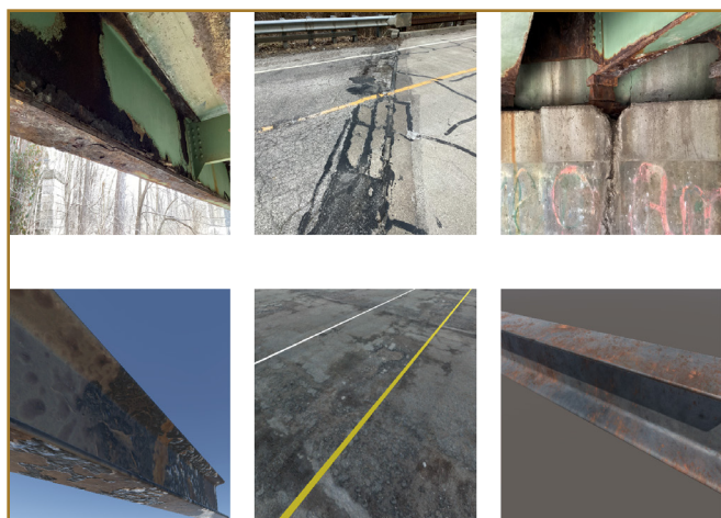
Representation of defects using synthetic modeling: heavy corrosion on steel beams and extensive cracking and spalling in concrete roads. (top) samples of real bridge components taken from Case Study 1 and (bottom) corresponding synthetic modeled recreations.
