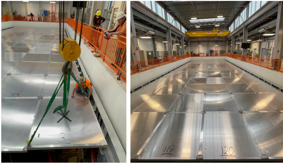
Figure 3.25: Left: details of the last installed Top CRT module. Right: picture of the fully installed Top CRT taken from the ground floor of the detector building.
