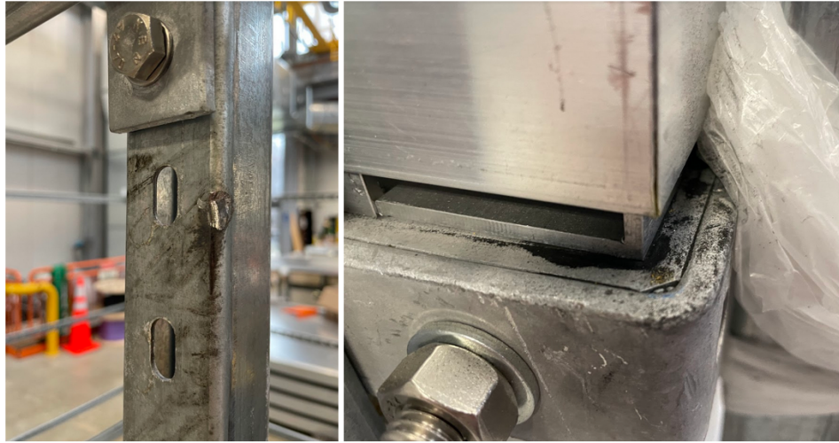
Figure 3.22: Left: detail of a dent found in one of the rack with malfunctioning modules. Right: details of black soot found on the CRT module supports of the rack.
