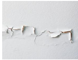
Crumbing plaster behind rain penetration
