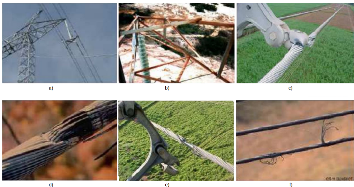
Figure 1.1 – Common faults in power transmission line structures (a) Loose wire structure, (b) Corroded structure, (c) Cable damaged by shock absorber, (d) Corroded cable, (e) Loose and damaged cable and (f) Broken cable.
