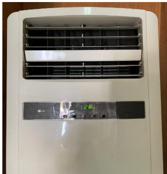
Figure 2. The condition of the Air Conditioner in the storage room
