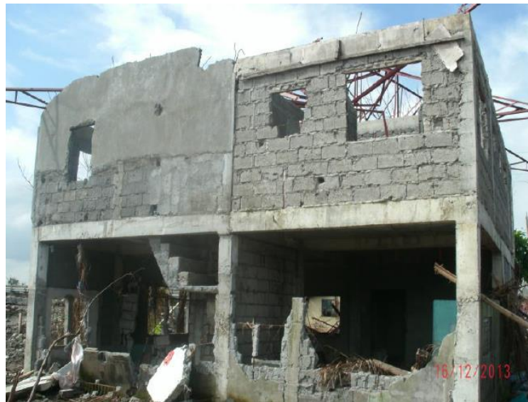
Figure 2. Damaged house in Palo, Leyte.
