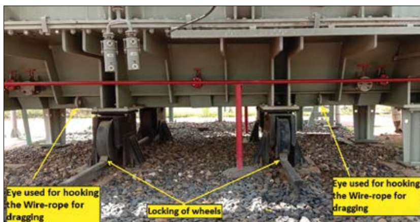
Figure 5. Wheels of the transformer are shown locked on rail pieces grouted on the plinth, and eyes are shown for hooking a wire-ropes for dragging
