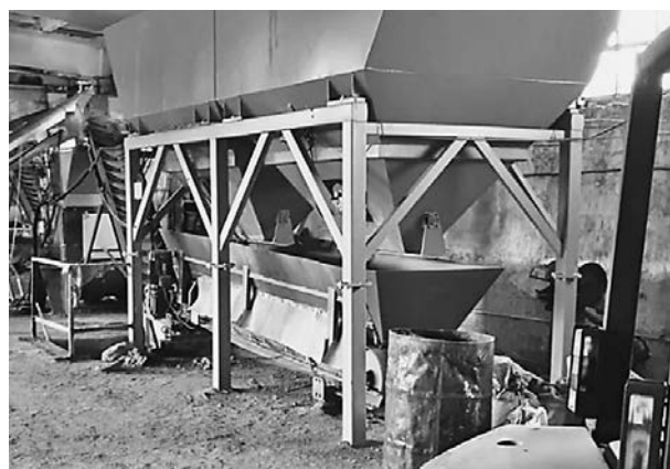
Figure 10 Vertical bins for bulk materials
