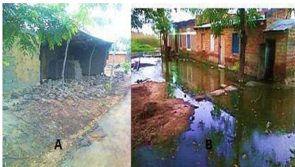
Photo A : a house collapsed in the Majengo district by torrential rain in June 2018 andphoto B : a flooded plot in the AEBAZ district in June 2018.
