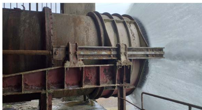
Fig 1. Hydraulic shock in the intake part of the Karkidon reservoir
