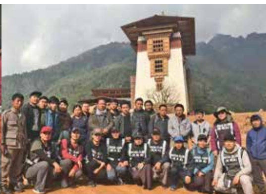
Voluntary labour contribution by RMA staff at Drukgyel Dzong re-construction at Paro on March 17, 2018.
