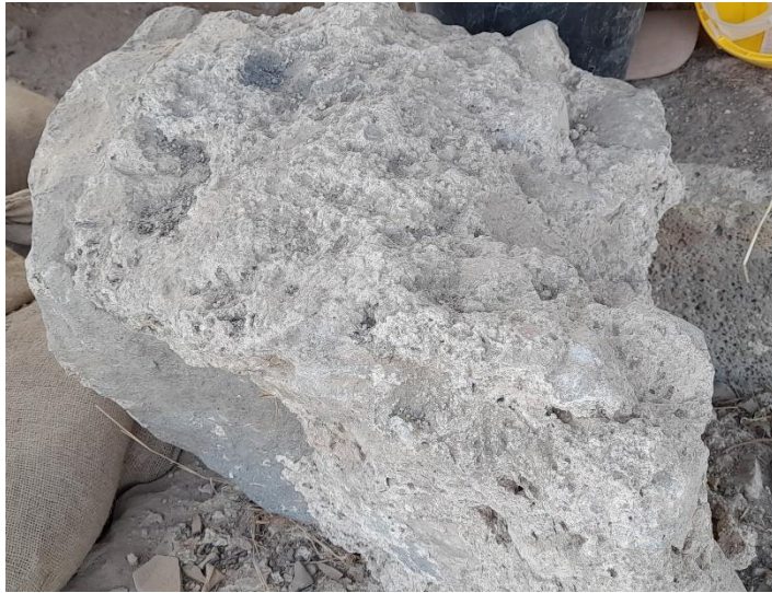
Figure 16. Fallen block from the W3003. (Photo by K. Thomas)
