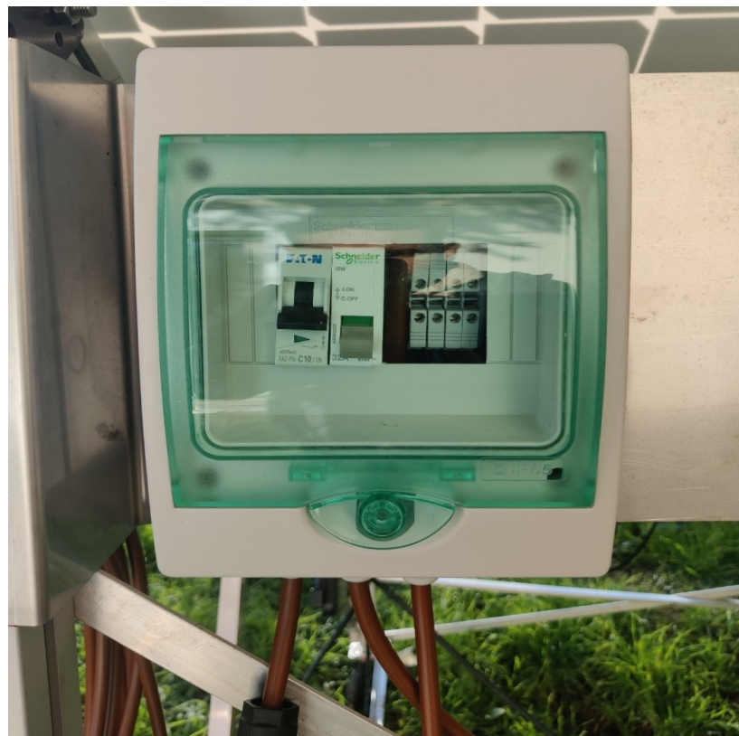
Figure 3.9 : Main power switch mounted on the back of half cut PV module structure
