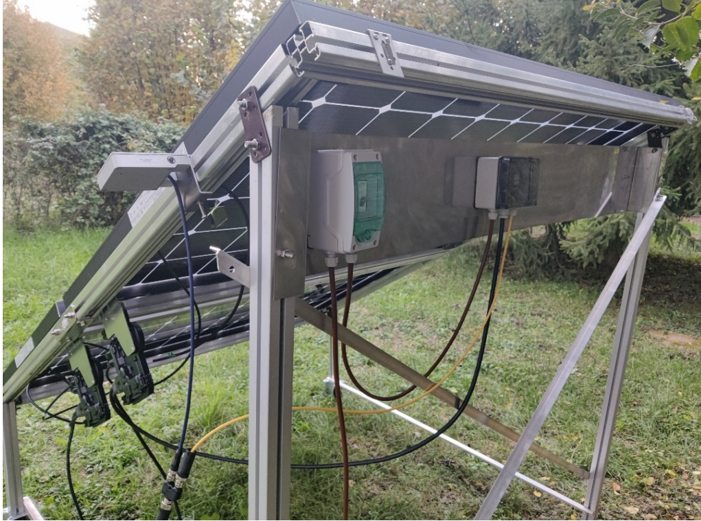
Figure 2.4 : Rear view of the experimental setup with the bifacial PV module
