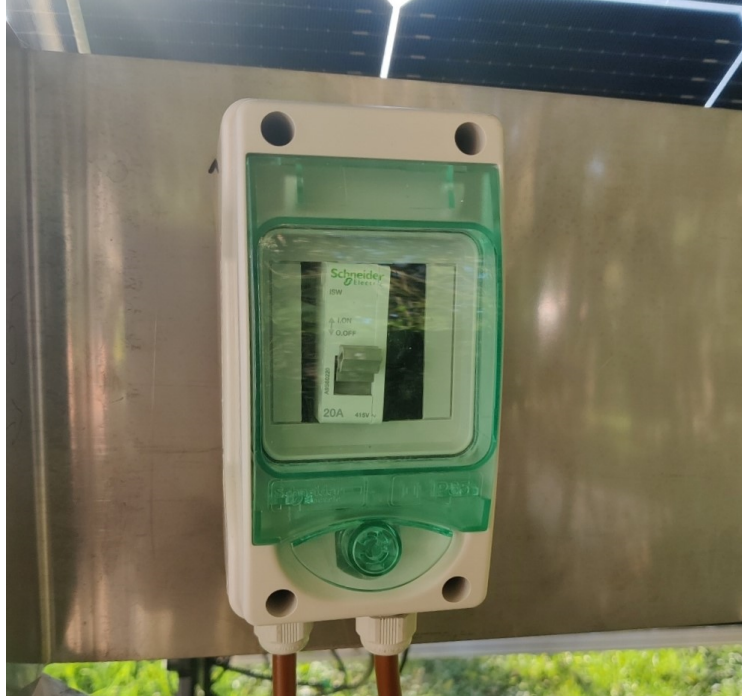
Figure 3.10 : Dedicated power switch mounted on the back of bifacial cut PV module structure
