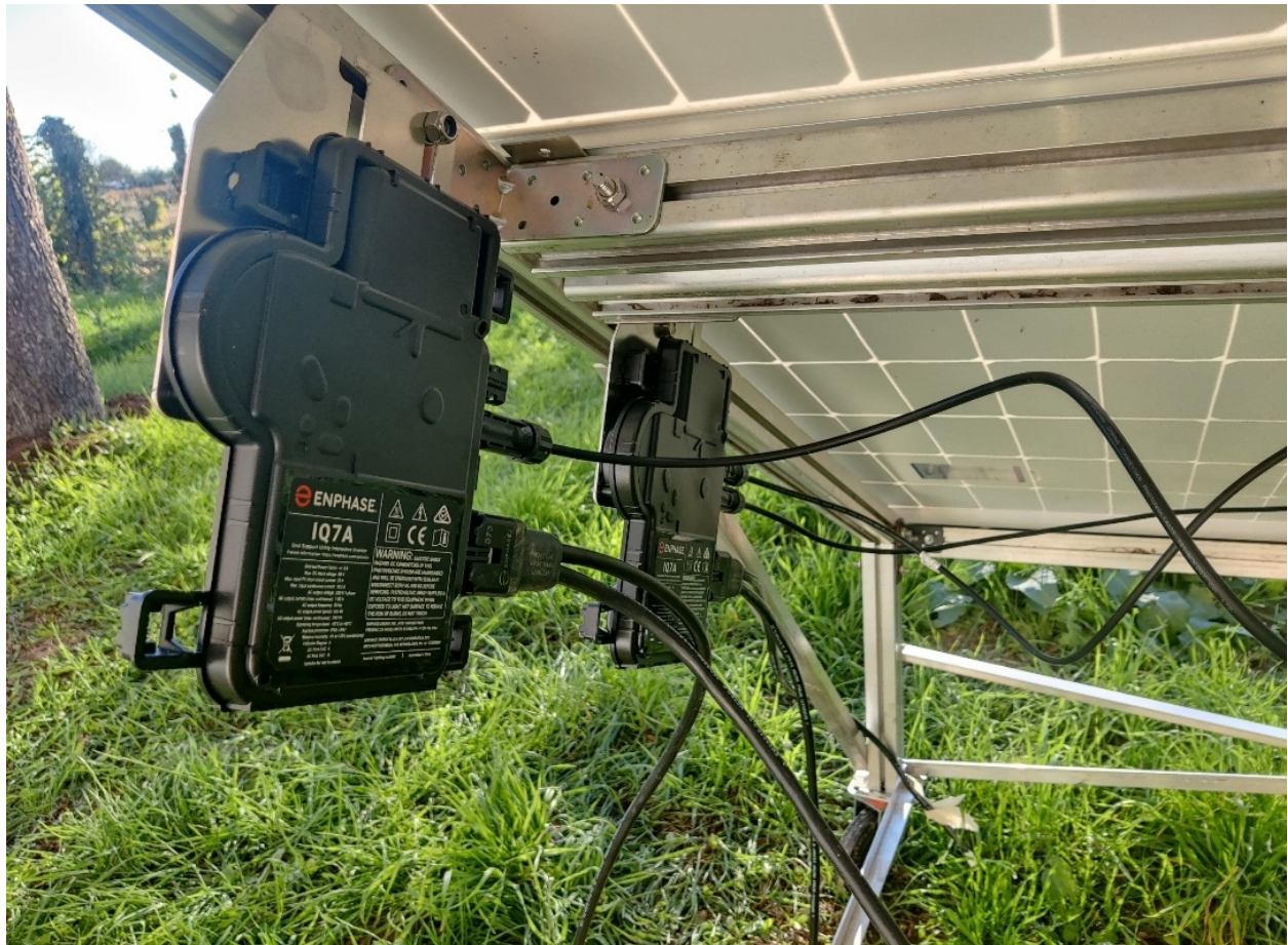
Figure 3.5 : Microinverter mounted under the half cut PV module structure
