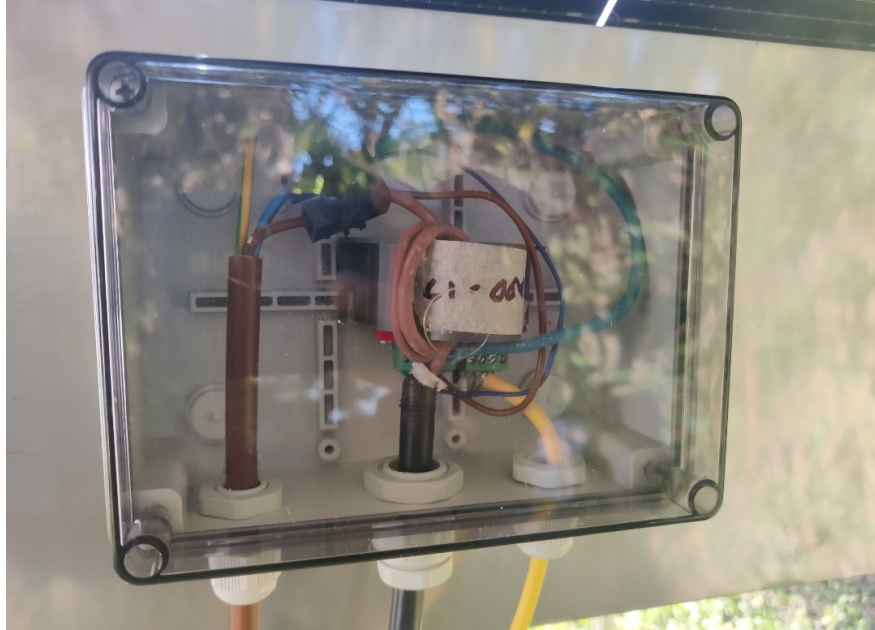
Figure 3.7 : Wattmeter mounted on the back of half cut PV module structure
