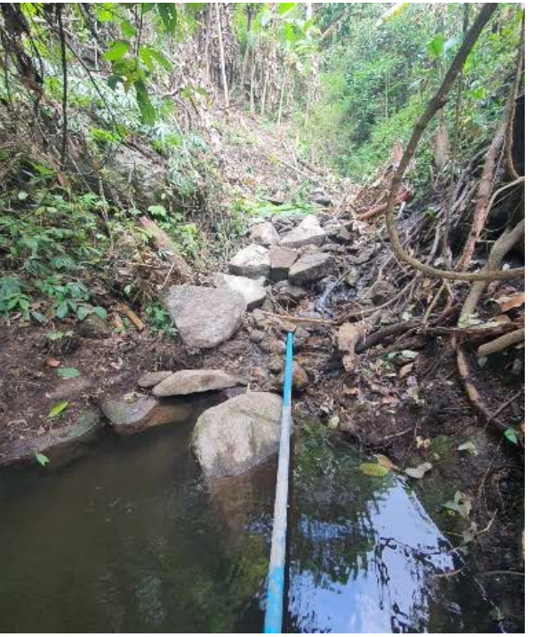
Figure 2 - Gravity-fed water system
