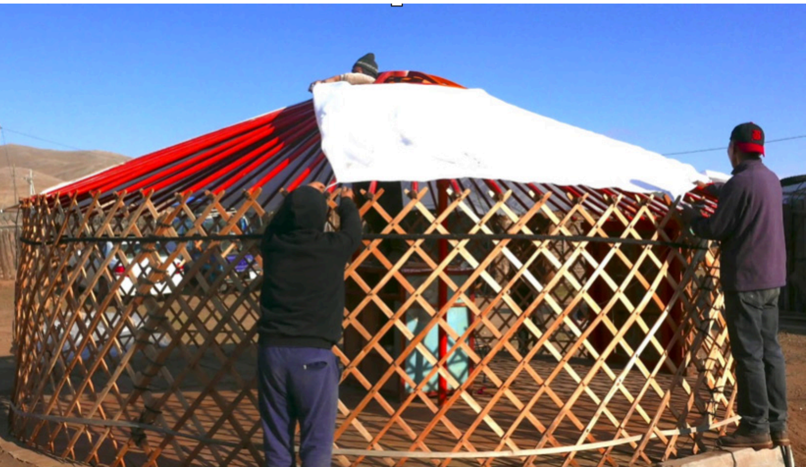
Figure 20: Wooden frames of the Mongolian yurts are made of wicker strips which is cross arranged to form a supporting structure composed of multiple diamond shapes (Youtube).
