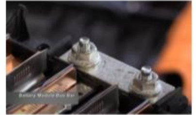
Connection of 2 adjacent module with bus bar -ve of one module to + of module another module. Similarly all are connected in series
