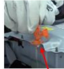
need the service grip to open the lock , insert and rotate to remind that there are high voltage under this cover
