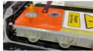
Brick is connected with base with side bolt 10 no and other side with mounting rail
