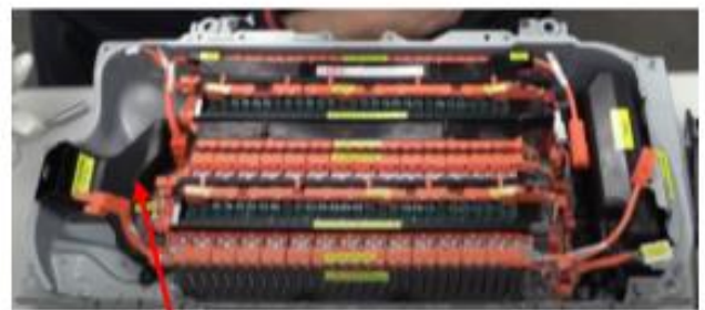
inlet duct split in two
