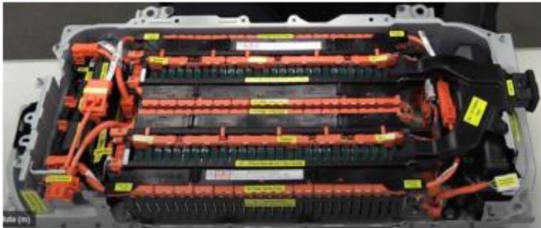
After removal of top cover
