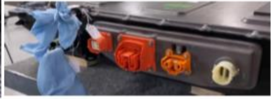
Front battery connection
