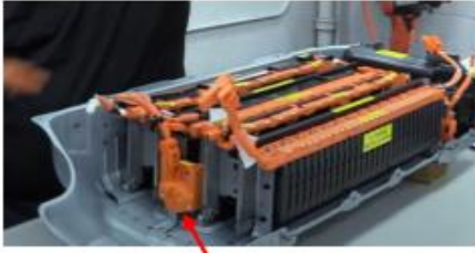
high voltage fuse, connected with +ve terminal one clip which holds the clamp, 125A Fuse
