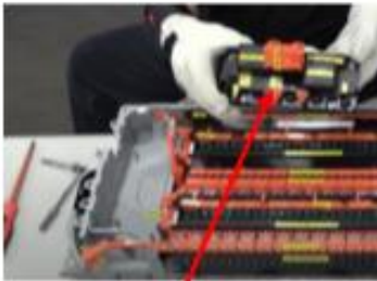
-ve contactor, +ve contactor, pre charge + contactor, current sensor, resistor, pre charge register,
