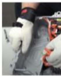
Junction box tray fixed with one bolt
