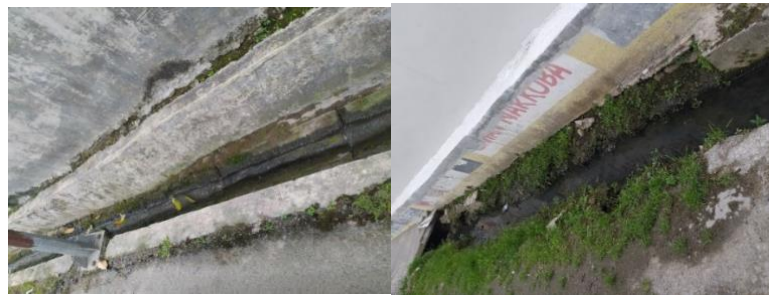
Figure 10. Drainage Conditions on Jalan Abadi (Left) and Jalan Sehat (Right) in Kecamatan Medan Sunggal
