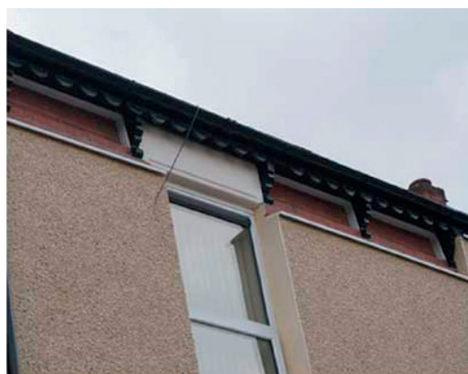
Figure 1: An illustration of a difficult detail in terms of external wall insulation 8
