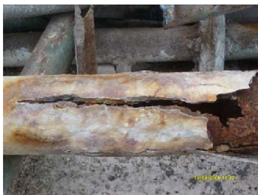
c) corrosion damage to pipelines
