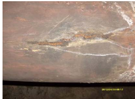
b) through cracks in the steam pipe
