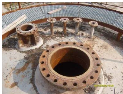
d) corrosion damage to the spherical tank
