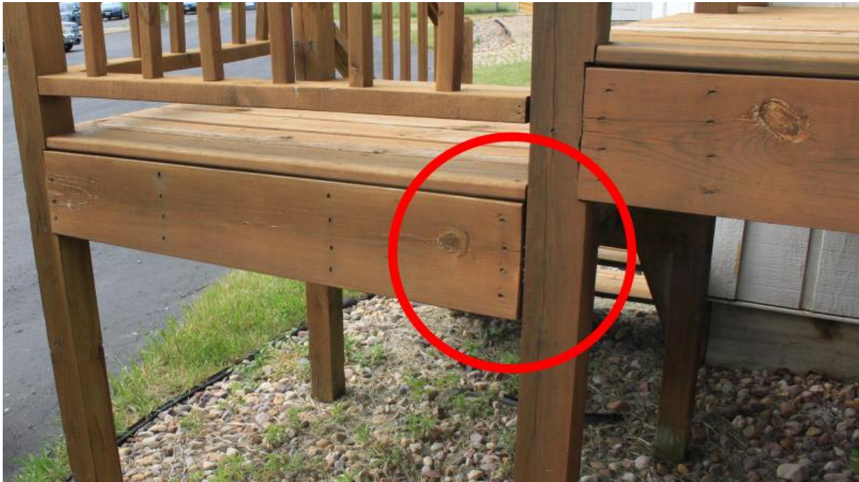
Figure 3 The circled image is the joist box and the rail. The circle is showing how the Joist box to rail connection is showing insufficient fixity.
