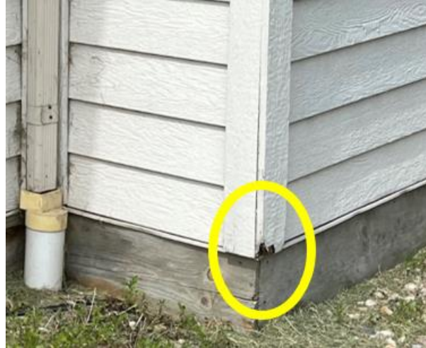
Figure 23 The image is of the trim boards of the house and the trim boards around the house are showing signs of decay due to failure of paint.
