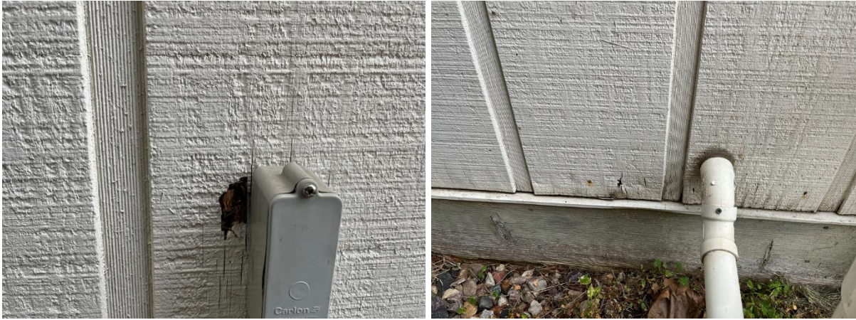
Figure 22 The photograph is of the areas where utilities are attached and show similar signs of decay.
