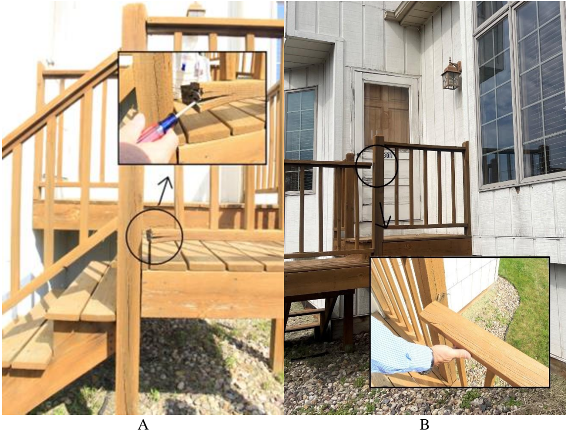
Figure 5 A and B, the images are of the back deck, and it shows the problematic areas. Images of the rail-to-post connects have completely failed in the highlighted location.
