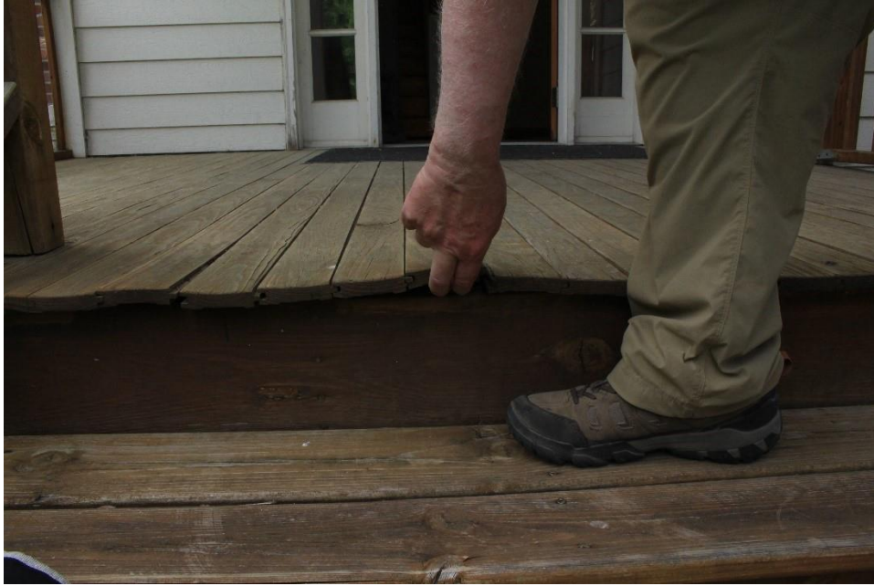
Figure 14 Dr. Ross is bending over to show where the front porch can be lifted, therefore, the porch flooring near the top of the steps has become unfastened due to fastener corrosion.
