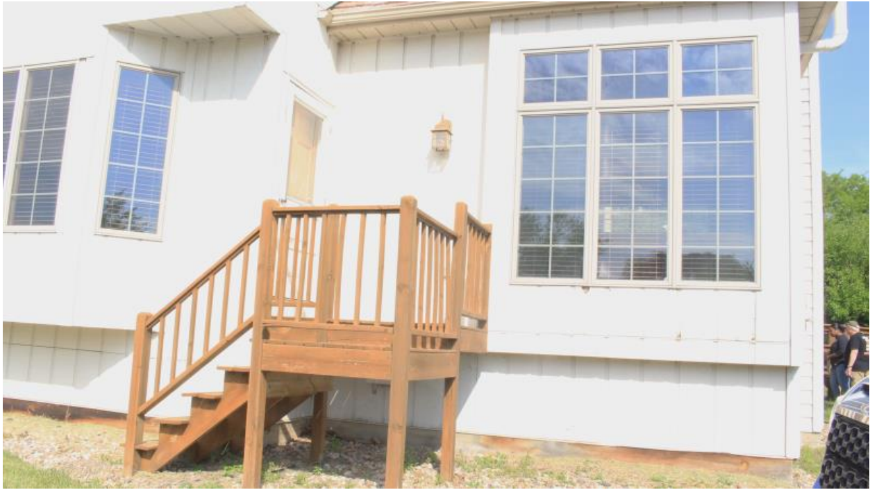
Figure 17 The image is the back deck of the demo house where the T1-11 siding is mostly located on the house and the image shows signs of decay and missing pieces of the siding.
