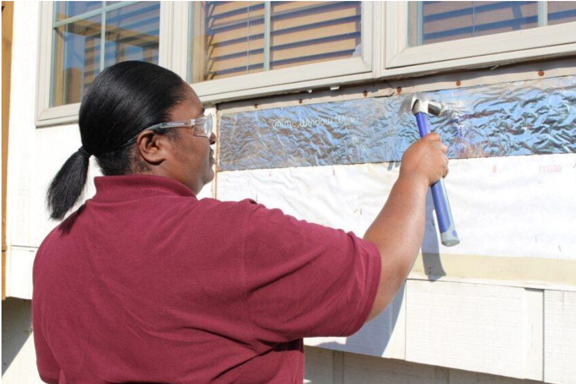
Figure 1 This image is illustrating the student using a hammer gently striking silver area which is the sheath underneath the siding of the house to determine if moisture is present.
