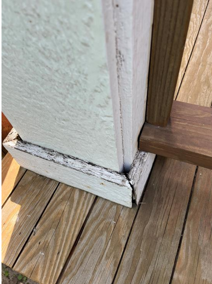
Figure 15 The image is still of the front porch entrance and the post trim showing signs of deterioration.
