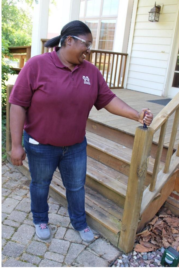
Figure 12 The student is inserting a flat head screwdriver into the post to indicate decay is present in the structure.
