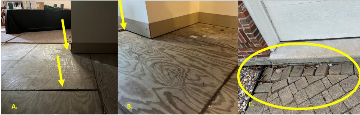
Figure 26 These images show signs of settling in the foundation, photo located in the southwest portion of the basement and top left photo in front of the carport. The treated plywood foundation shows un-leveling underneath the flooring.
