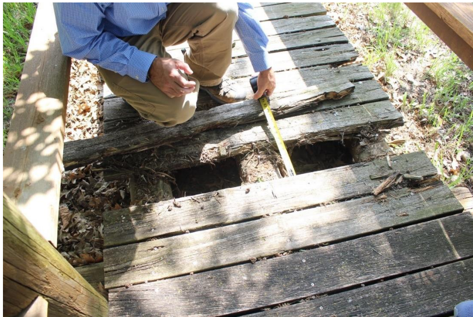
Figure 7 Dr. Shmulsky is measuring the deteriorated area with a tape measurer to get the width of the deteriorated deck that was removed. Some of the deck could be removed without effort as illustrated in the image above.
