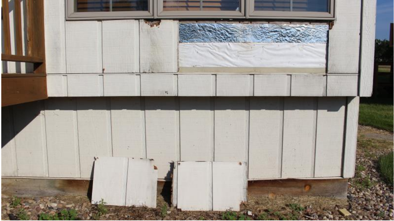
Figure 20 This image shows the section of T1-11 siding removed beneath the triple mullion dining room window to prepare to test the silver area to indicating if moisture is present behind the siding.
