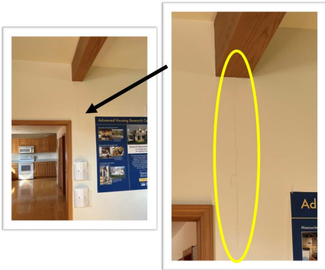
Figure 25 A fracture or buckling of sheet rock in the great room and the right-side header inside the great room shows fracture or buckling in the drywall above the door opening.
