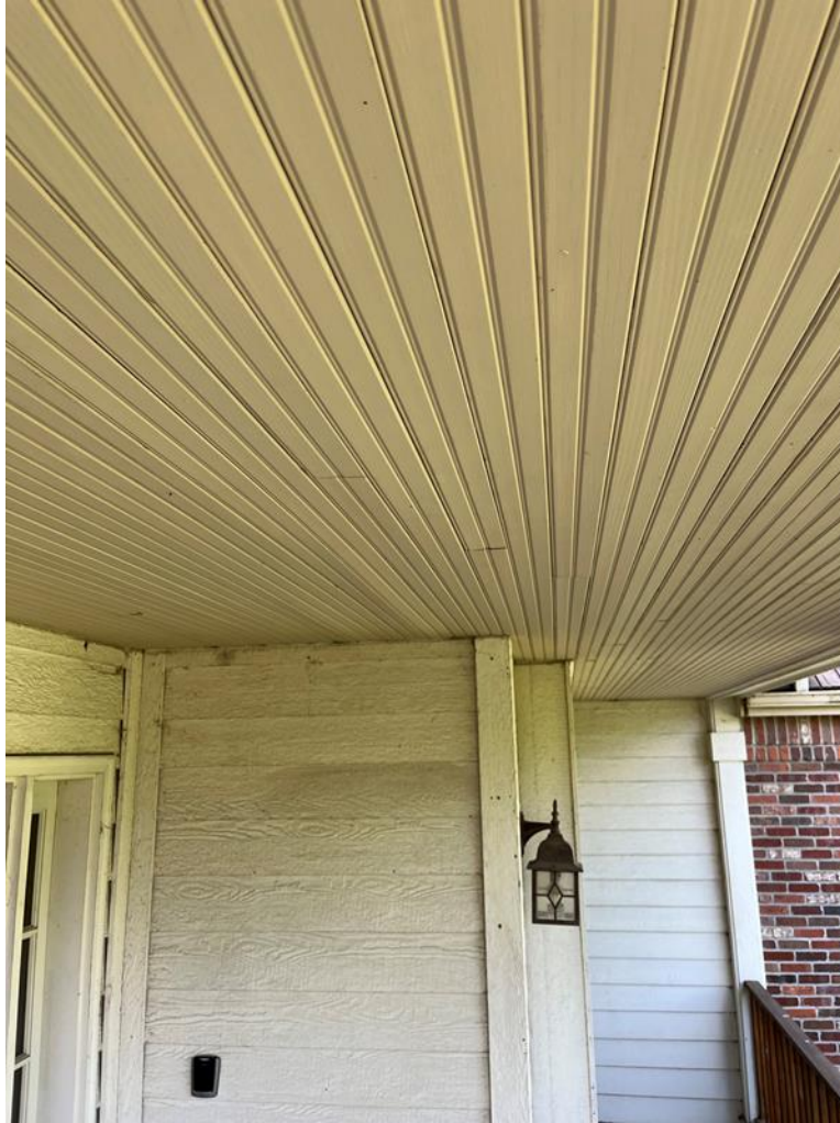
Figure 16 The image is of the front porch ceiling, and the photo depicts tongue and groove ceiling swelling indicating moisture issues.
