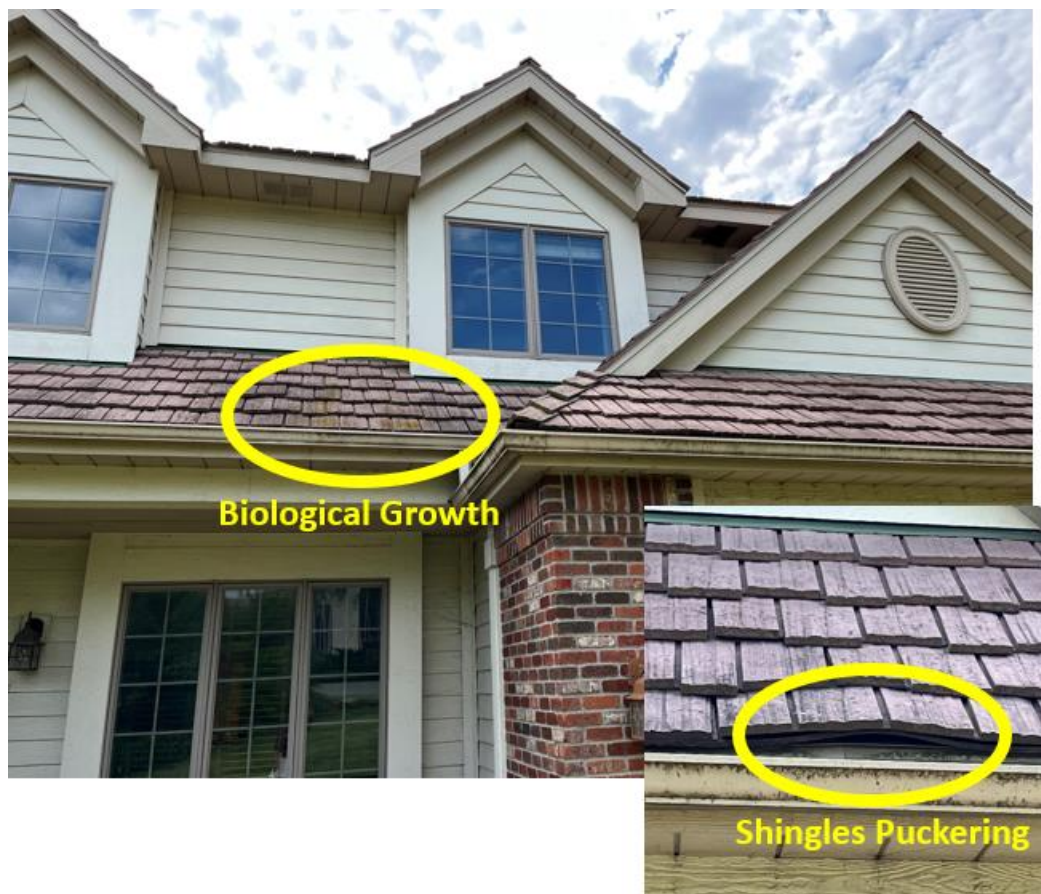
Figure 24 The image is of the roof shingles and the shingles showing signs of weathering. Biological growth and puckering can be seen on the shingles of the roof.
