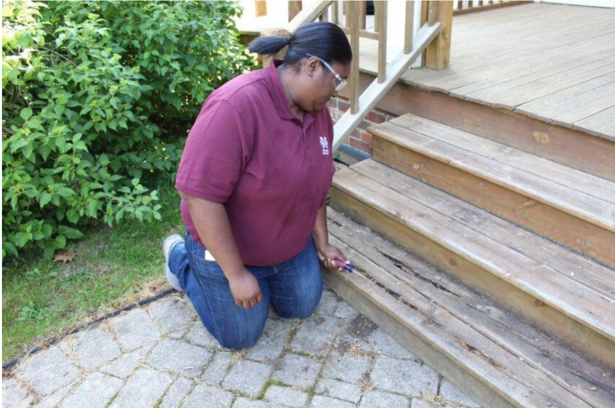
Figure 2 The student is kneeling down to insert a screwdriver into the front porch steps to measure the dept of decay.
