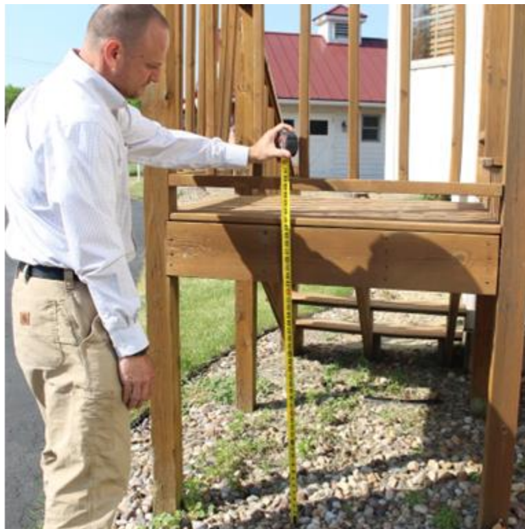
Figure 4 Dr. Shmulsky is measuring the deck height to ensure it is up to code with the International Residential Code.
