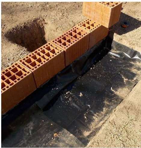
FIG. 8 GEOMEMBRANE BARRIER EXECUTED WITH POLYVINYL CHLORIDE (PVC) INSERTED INTO THE WALL AND AT 0.20M DEEP
