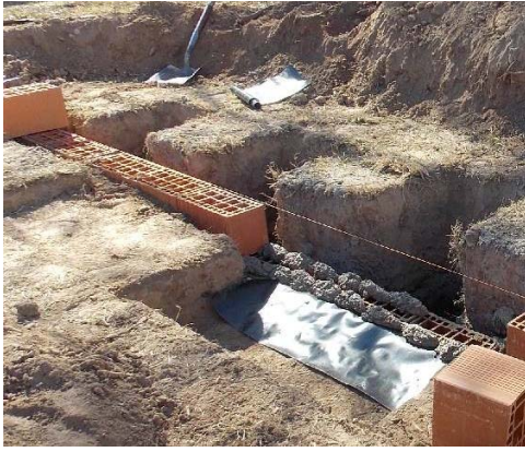
FIG. 7 CONSTRUCTION OF SOIL-BENTONITE BARRIER. PLACEMENT OF POLYETHYLENE FILM TO SEAL JOINT BETWEEN WALL AND BARRIER
