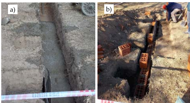
FIG. 5 IMAGES OF THE CONSTRUCTION OF THE PHYSICAL MODEL. A) FOUNDATION CONSTRUCTION. B) LAYING CERAMIC BLOCKS.
