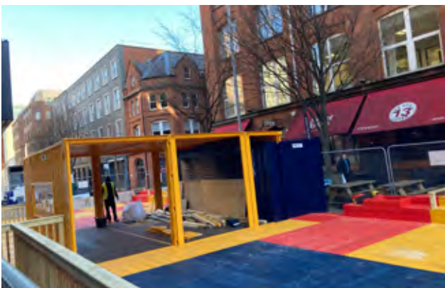
Figure 73: Brunswick Social, in progress images from Brunswick Street to new container hospitality unit (Authors, March 2022)
