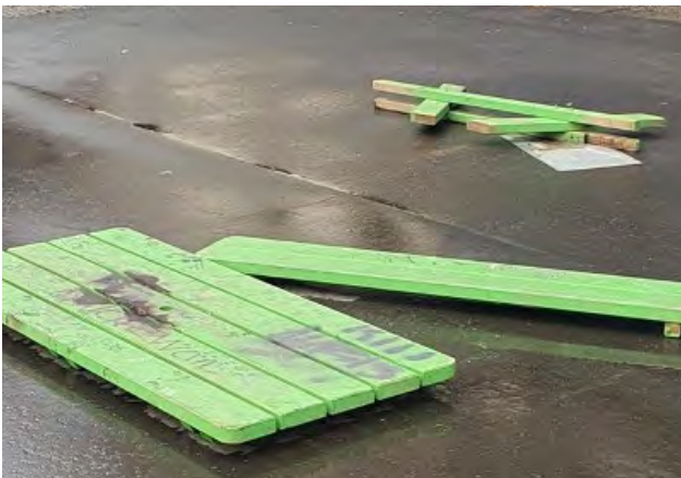
Figure 39: Cathedral Gardens - vandalism, fire damage to artificial surface (Golden, July 2021; CQ Belfast, 2022)
