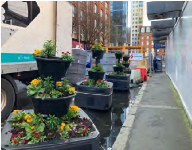
Figure 77: Brunswick Street Social, in-progress construction with access and servicing at Travelodge Hotel (Authors, March 2022)
