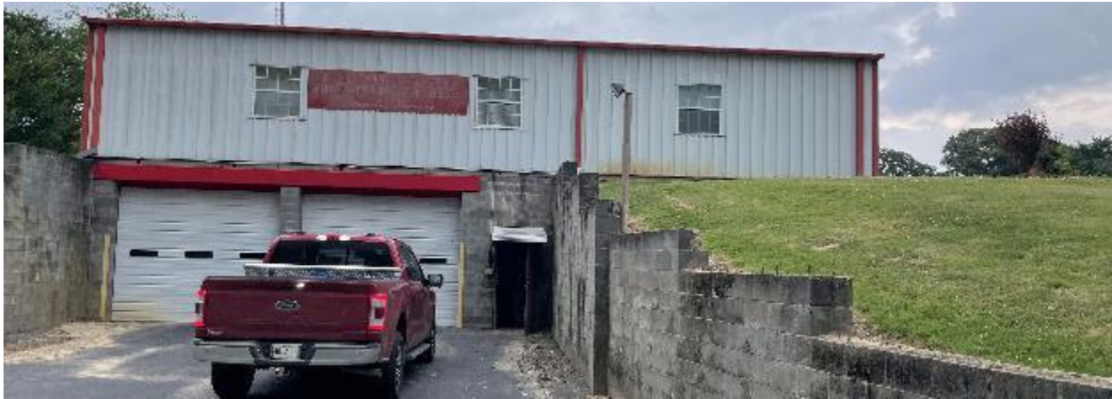
Figure 3.21 Soft Story Vertical Irregularity from Site Visit
