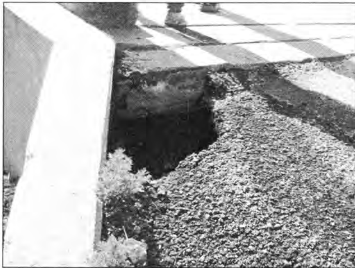
Figure 3.68 - Failure at the Approach Slab Shoulder (Bridge No. 7821.1L680 - WBL)
