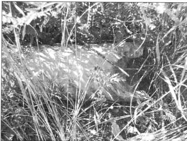
Figure 3.250 - Damaged End Drain Outlet (Bridge No. 7781.2065 - North End of NBL)
