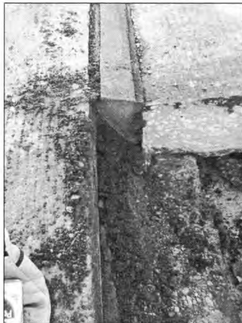
Figure 3. 35 - Flexible Foam Used to Seal the Expansion Joint (Bridge Carrying 160 over I-35)
