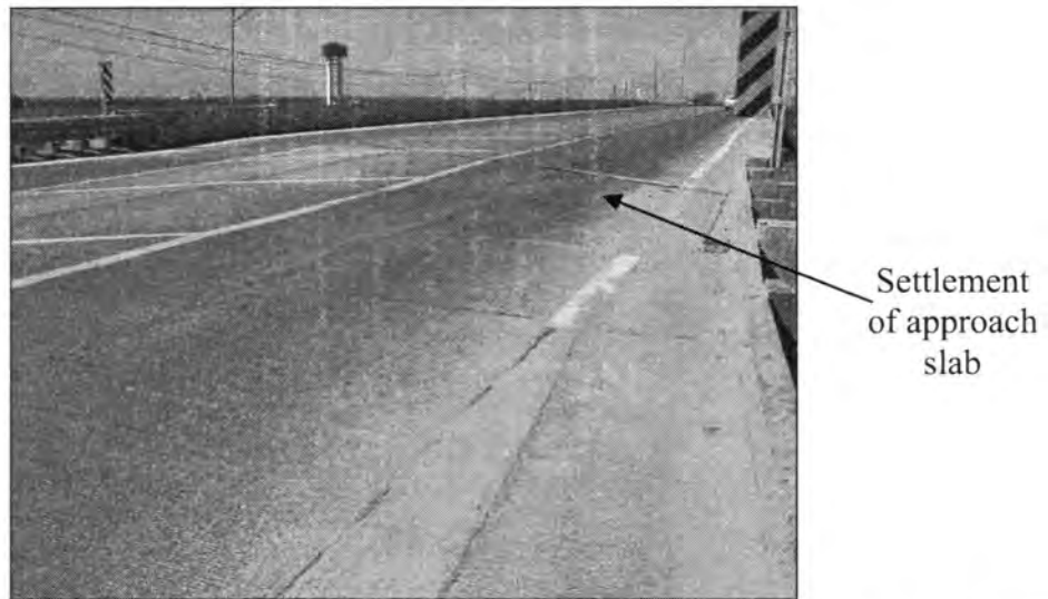
Figure 3.79 - Differential Settlement at the Bridge Approach (Bridge at Clay St. Crossing I-35 - East End)
