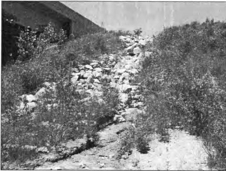
Figure 3. 172 - Rocks Placed at the Abutment Side to Prevent Erosion (Bridge No. 76.8065 - North End of NBL)
