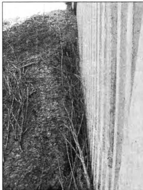
Figure 3.82 - Erosion Along the Abutment Side (Bridge at Clay St. Crossing I-35 - East End)
