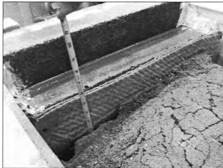
Figure 3.310 - Void Developed under the Approach Slab
