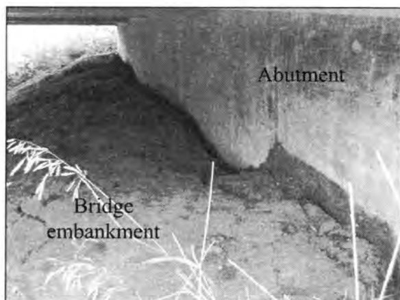
(a) Erosion at the Bridge Embankment
