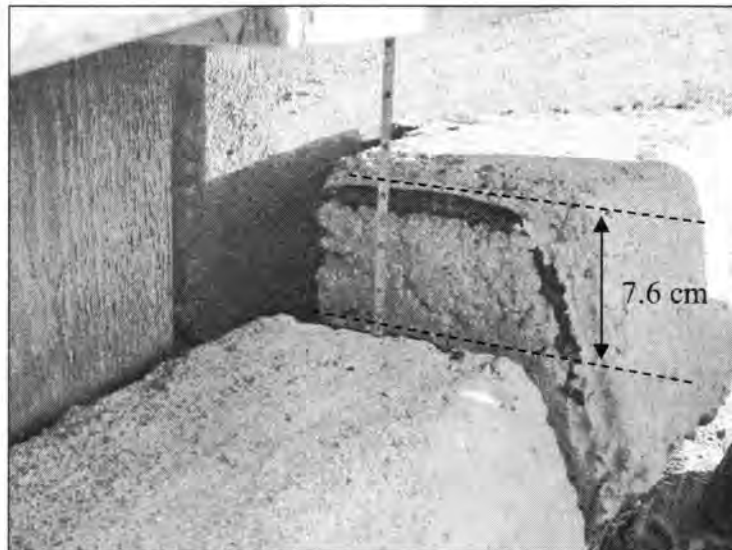
Figure 3.97 - Differential Settlement at the Bridge Approach (Bridge No. 574.2S001 - SBL)
