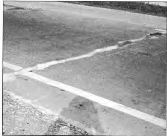
(b) Closer Image of Faulted Approach Slab
