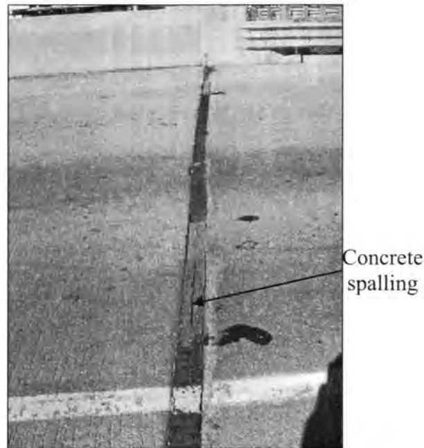
Figure 3.189 - Poorly Sealed Expansion Joint with Concrete Spalling (Bridge No. 1783.6018 - East End of EBL)
