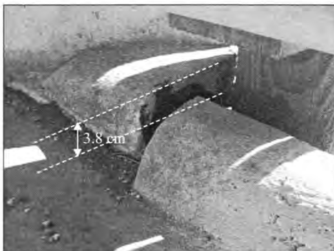
Figure 3.184 - Differential Settlement between the Bridge Approach and the Approach Slab (Bridge No. 1783.6018 - West End of EBL)
