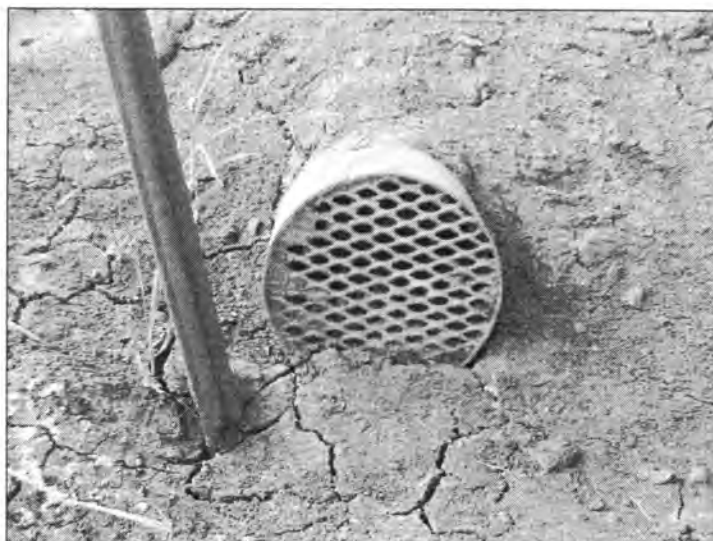
Figure 3.87 - "Wet-Drain" Filled with Soil Particles (Bridge at U.S. 218 over South Skunk River - South End of SBL)
