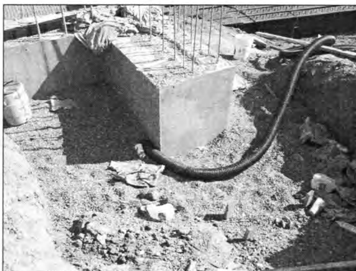
Figure 3.161 - Constructed Bridge Backwall with Visible Subdrain Surrounded by Porous Backfill (Euclid Avenue Bridge)
