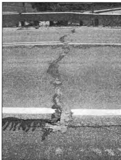
Figure 3.24 - Transverse Cracks of Recently Resurfaced Approach Slab (Bridge Carrying 72 nd St. over I-35 - East End)
