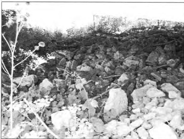
Figure 3.173 - Rocks Placed at the Bridge Embankment to Prevent Further Erosion (Bridge No. 76.8065 - South End of NBL)
