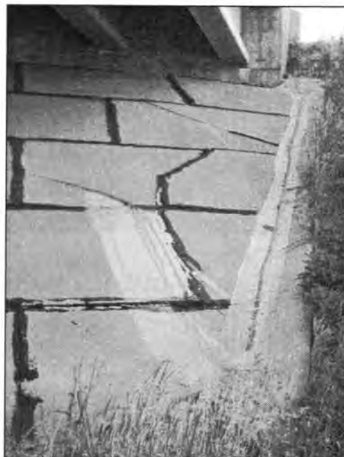
Figure 3.106 - Cracking of the Slope Protection (Bridge No. 574.2S001)
