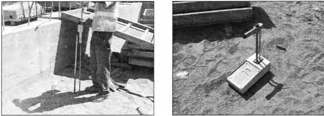
Figure 3.137 - DCP and Nuclear Gauge Tests (Polk Blvd. Bridge - North End of NBL)
