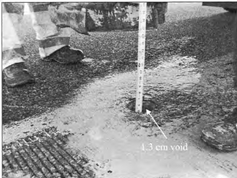
Figure 3.254 - Measuring the Void under the Approach Slab (Bridge No. 7781.2065 - North End of SBL)
