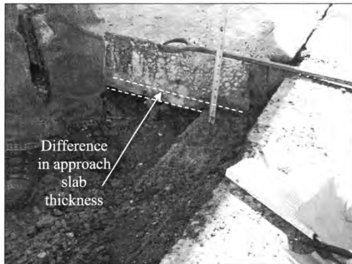
Figure 3. 34 - Non Uniform Approach Slab thickness with 3.8 cm Increase Over the Backfill Compared with the Thickness over the Paving Notch (Bridge Carrying 160 over I-35)
