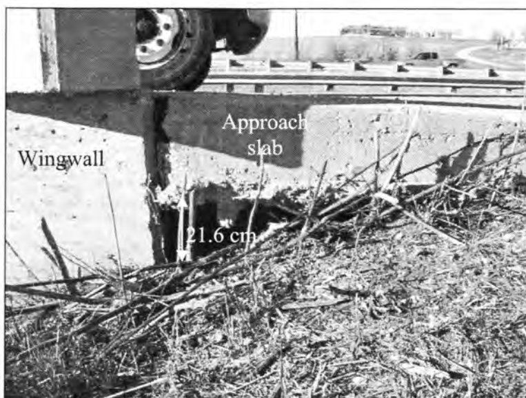
Figure 3.191 - Void under the Approach Slab (Bridge No. 7773.0R065 - North End of SBL)
