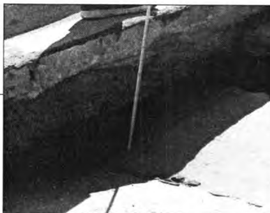
(b) Closer Image of the Damaged Concrete
