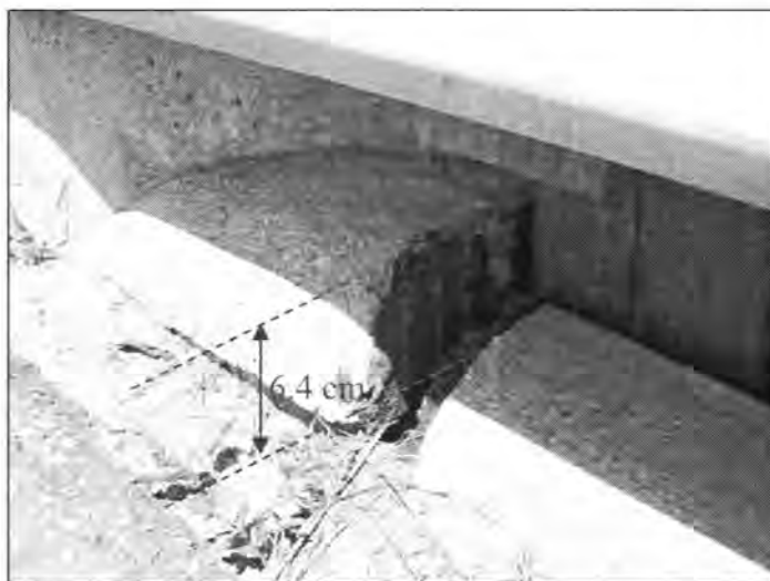
Figure 3.238 - Differential Settlement (Bridge No. 7779.4065 - South End of NBL)
