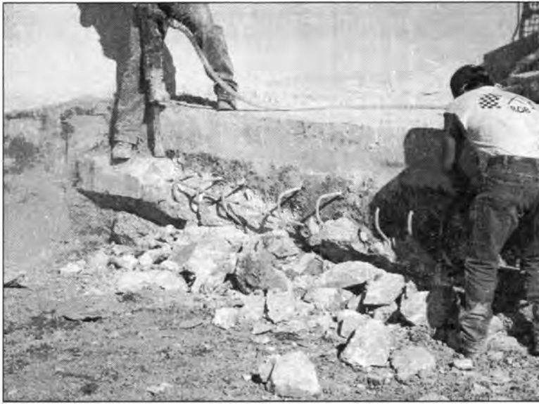
Figure 3.233 - Tearing Down the Old Pavement Notch (Bridge No. 7779.0065 - South End of SBL)
