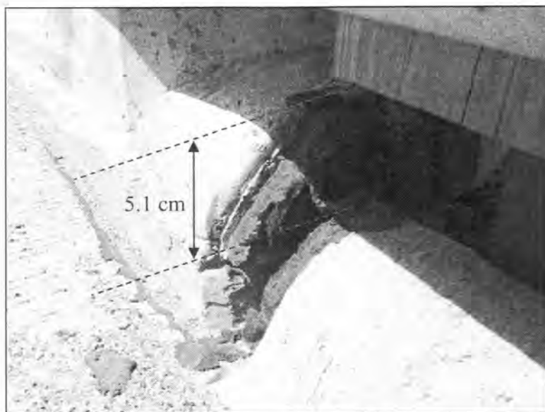
Figure 3.252 - Differential Settlement at the Bridge Approach (Bridge No. 7781.2065 - South End of NBL)
