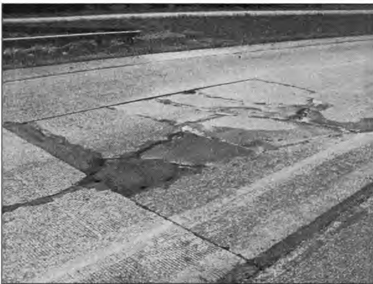
Figure 3.249 - Severe Cracking at the Bridge Approach Pavement (Bridge No. 7781.2065 - North End of NBL)
