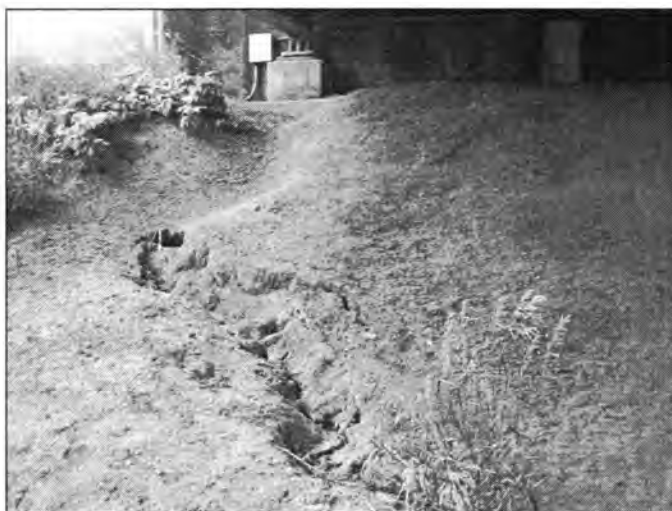
Figure 3.88 - Erosion of the Bridge Embankment (Bridge at U.S. 218 over South Skunk River - North End of NBL)
