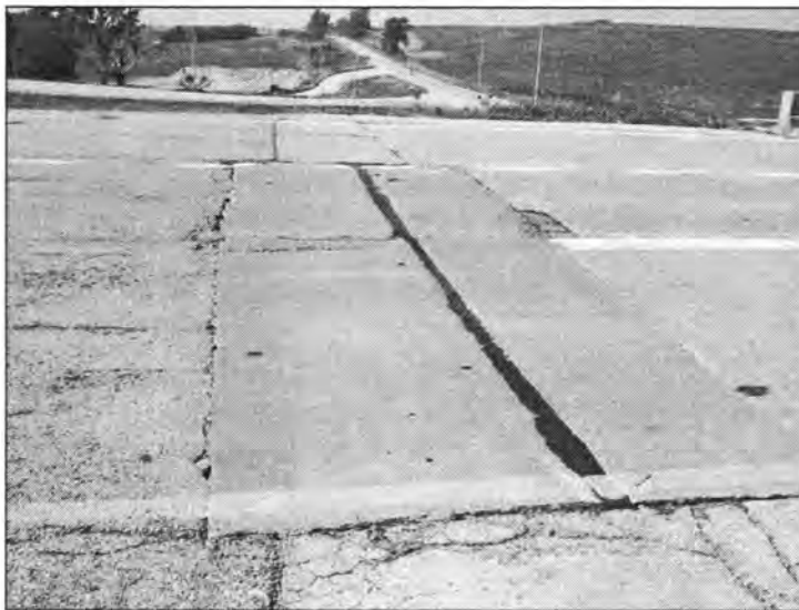
Figure 3.69 - Various Cracking at the Bridge Approach (Bridge No. 7821.1L680 - EBL)
