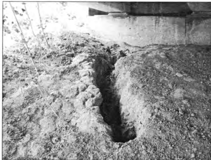
Figure 3.57 - Soil Erosion of the Bridge Embankment (Bridge No. 99)
