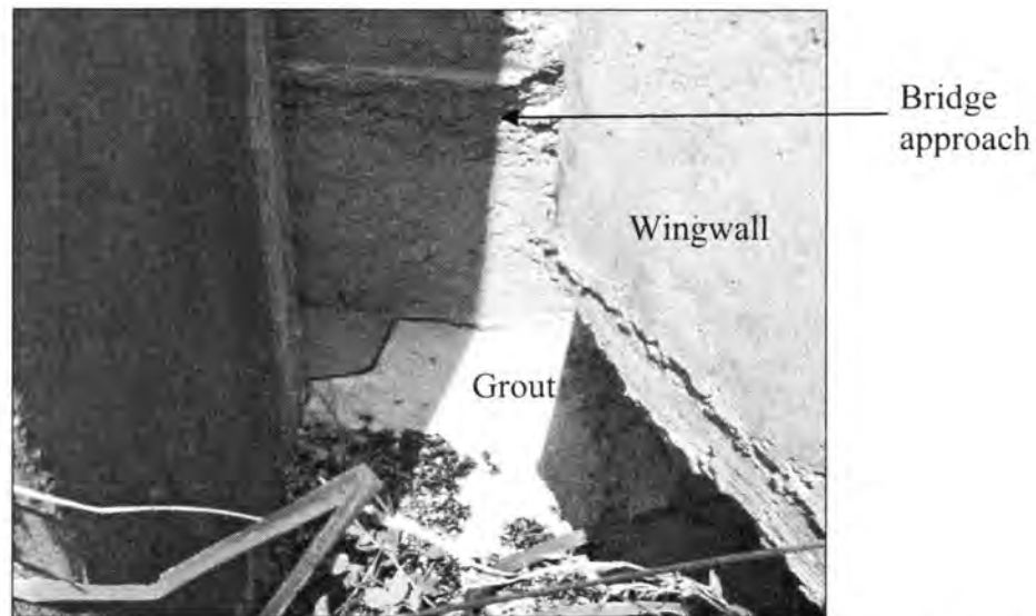
Figure 3.90 - Grouting Under the Approach Slab (Bridge at U.S. 218 - South End of NBL)
