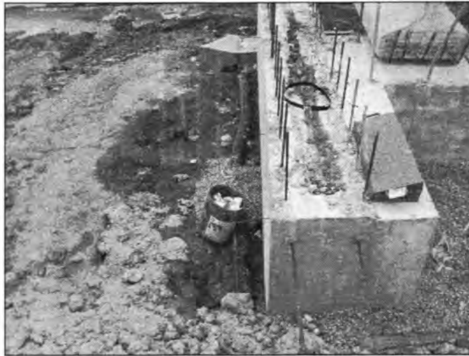
Figure 3.122 - Subdrain Placed Along the Side of the Abutment (35 th Street over I-235)
