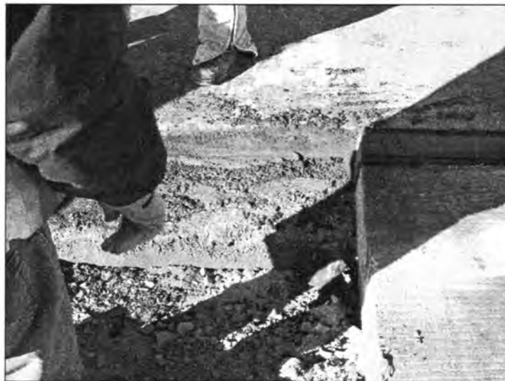
Figure 3.33 - Layer of Crushed Aggregate Covering the Paving Notch (Bridge Carrying 160 over I-35)
