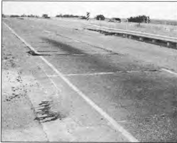
(a) Cracked Approach Slab Panels
