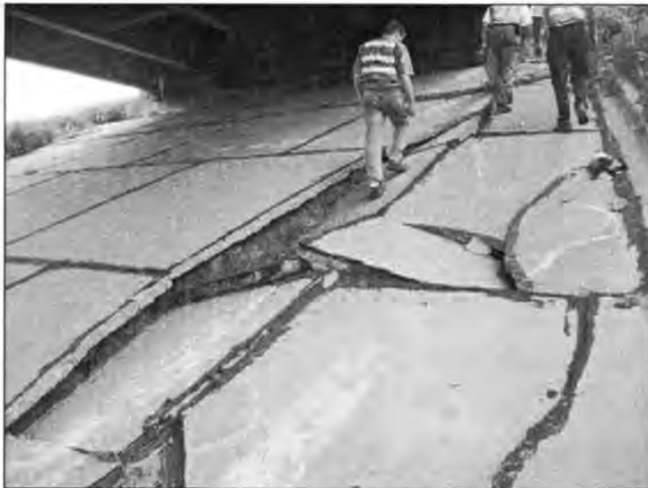
Figure 3.112 - Severe Damage of Concrete Slope Protection Due to Erosion (Bridge No. 5200.8R380)
