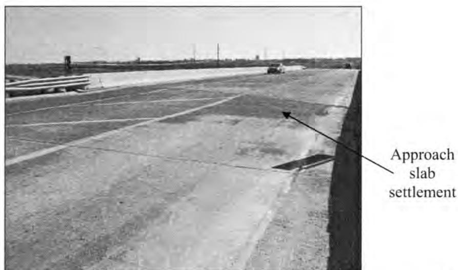
Figure 3. 75 - Settlement of the Approach Slab (Bridge at Clay St. Crossing I-35)
