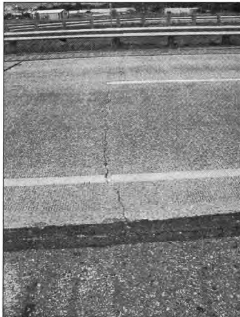
Figure 3.259 - Transverse Cracking at the Bridge Approach (Bridge No. 7782.8L065 - North End of SBL)
