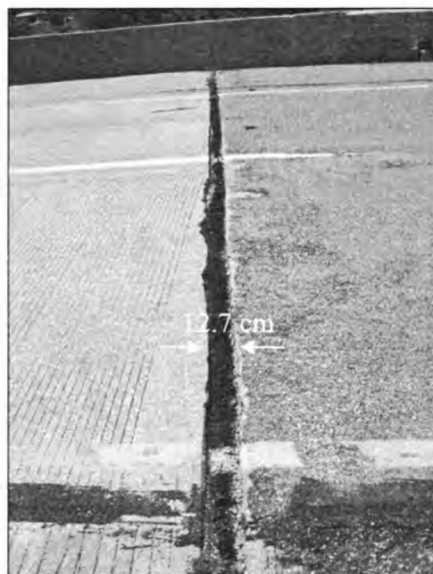
Figure 3.242 - Recycled Tires used as Joint Filler (Bridge No. 7779.4065)
