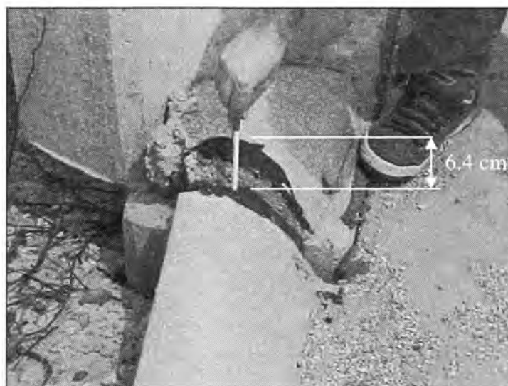
Figure 3.6 - Differential Settlement between the Bridge Deck and the Approach Slab (Bridge at U.S. 65 over South Skunk River - South End SBL)
