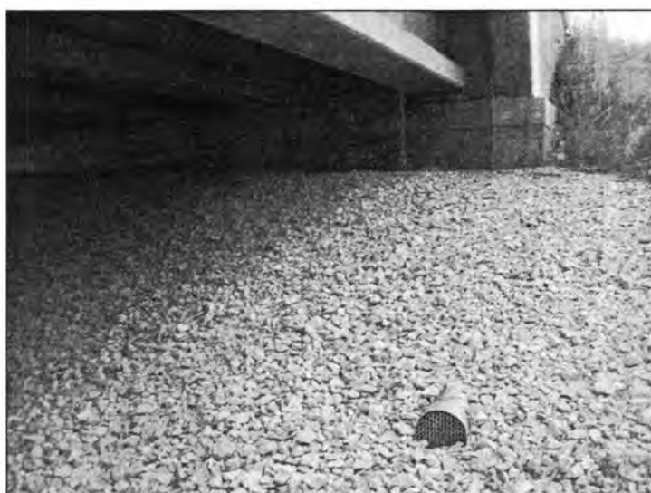
Figure 3.22 - Aggregate Used as a Slope Protection at the Bridge Embankment (Bridge Carrying 72 nd St. over I-35)
