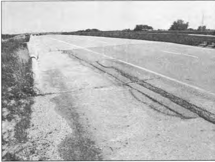
Figure 3.263 - Asphalt Overlay Placed Over the Approach Slab to Compensate for the Differential Settlement (Bridge No. 7783.1065 - North of End NBL)
