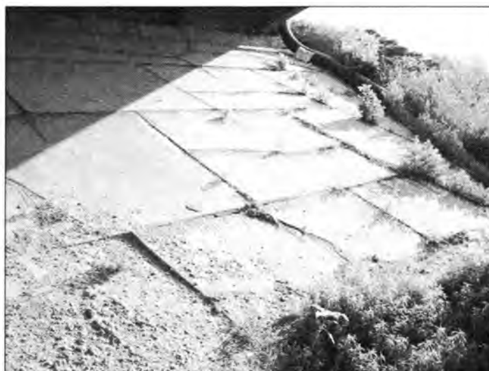
Figure 3.67 - Cracking of Concrete Slope Protection (Bridge No. 788.5R080)
