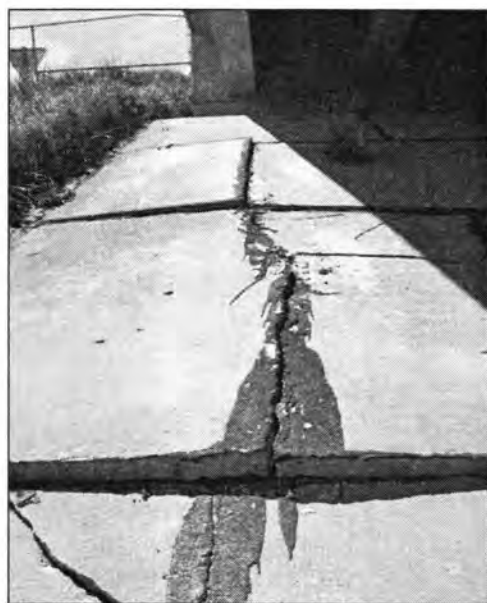
Figure 3. 46 - Fractured Concrete Slope Protection (Bridge No. 1793.6R035)
