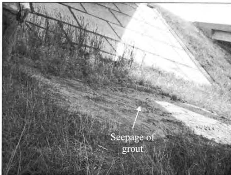
Figure 3.100 - Grout Seeping from the Bottom of the Embankment (Bridge No. 574.2S001)
