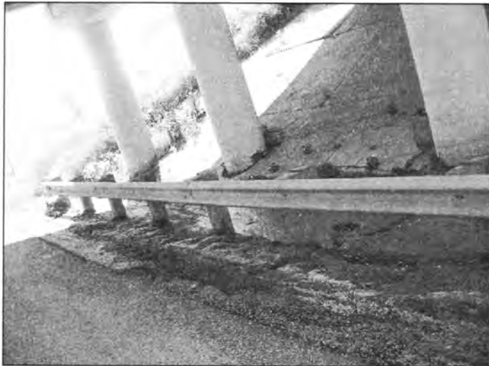
Figure 3.74 - Water Observed at the Bottom of the Embankment (Bridge No. 78071.5R29)
