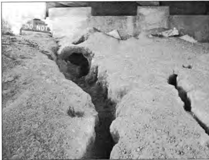
Figure 3.56 - Severe Erosion under the Bridge (Bridge No. 982.9)
