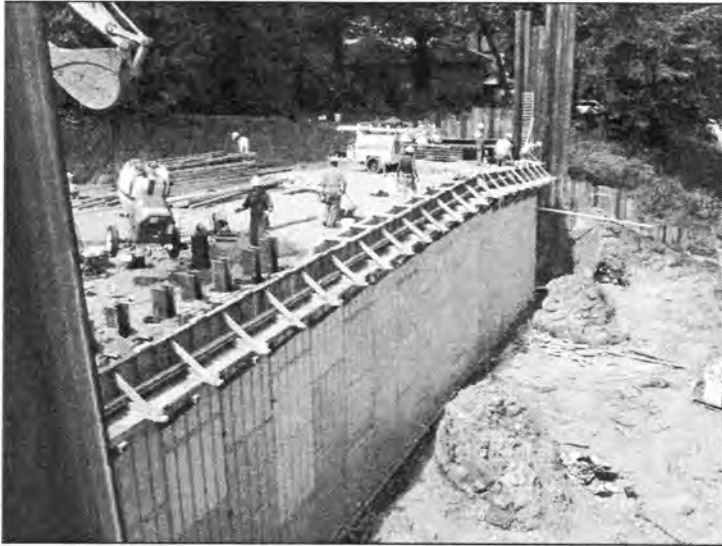
Figure 3.131 - Construction of the Retaining Wall (Polk Blvd. Bridge - South End of NBL)
