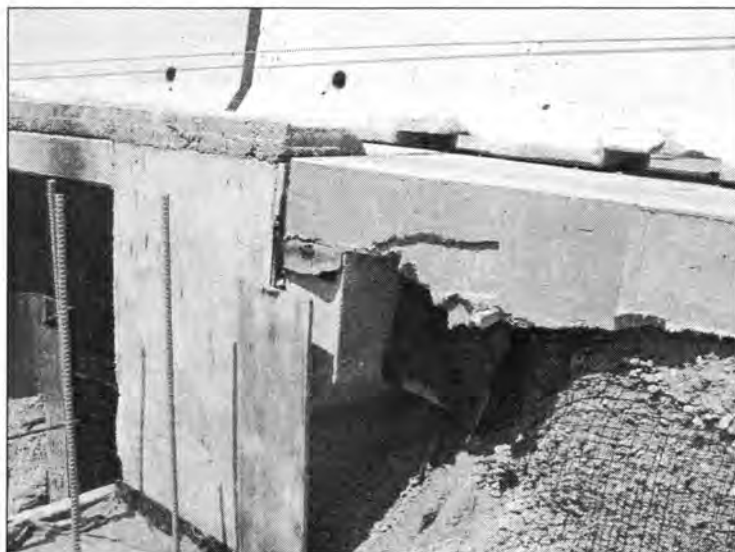
Figure 3.160 - A Closer Image of the Poorly Placed Granular Backfill (Euclid Avenue Bridge - NBL)
