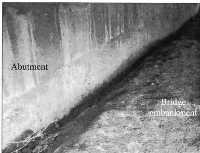
Figure 3.93 - Erosion of the Embankment Soil (Bridge No. 9266.2R - West End of WBL)
