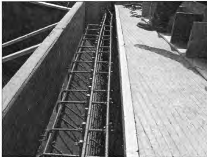
Figure 3.171 - Abutment Reinforcement (Bridge at U.S. 218 Crossing Rail Road - North End of NBL)
