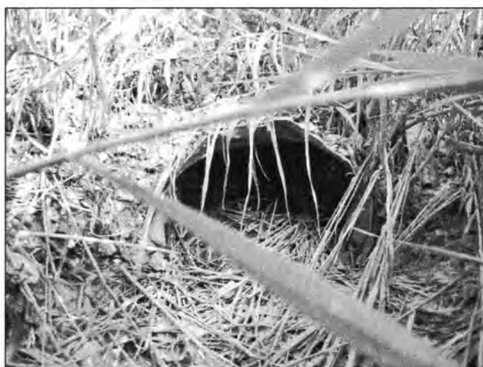
Figure 3.64 - End Drain Plugged with Soil (Bridge No. 786.8R080)
