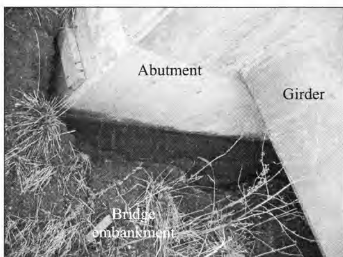
Figure 3.39 - Water Ponding on the Embankment under the Bridge (Bridge No. 1270.2S014)
