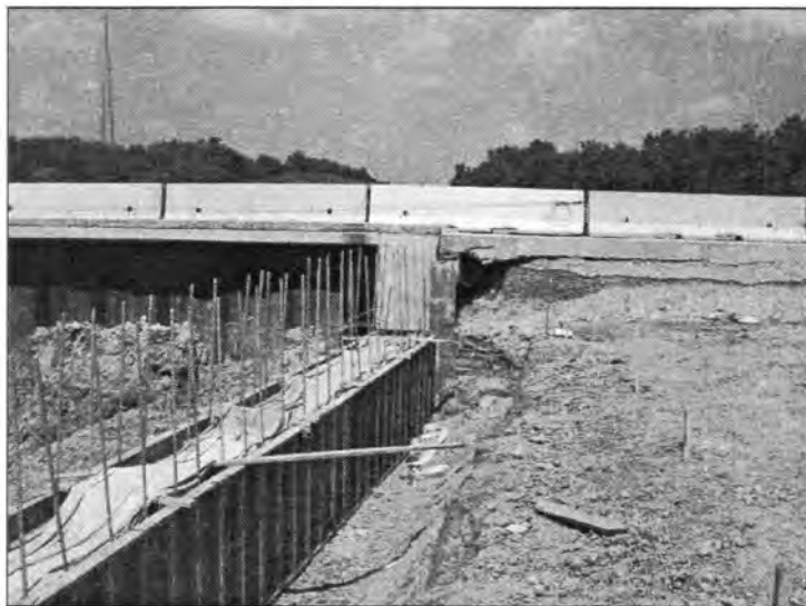
Figure 3.159 - Abutment Reinforcement and Backfill Placed at the North Bound Lane Approach Slab (Euclid Avenue Bridge)
