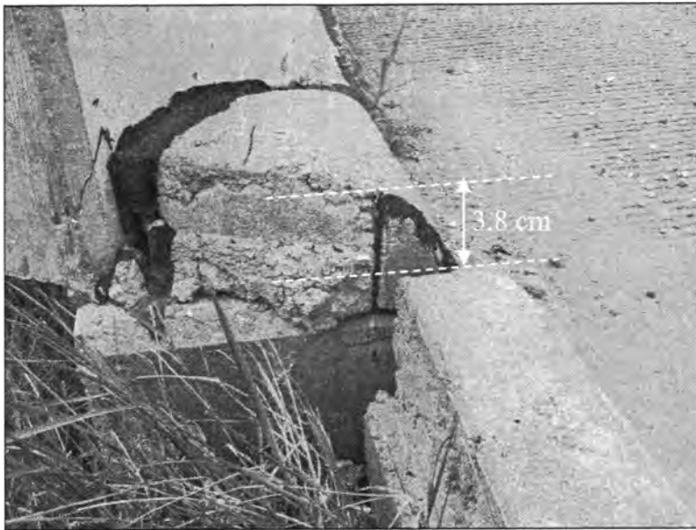
Figure 3.227 - Differential Settlement between the Bridge Deck and the Bridge Approach (Bridge No. 7779.0065 - North End of NBL)
