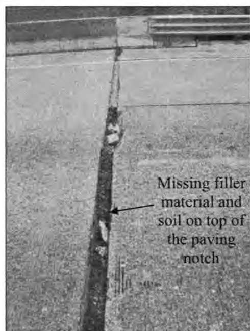
Figure 3.95 - Missing Filler Material Exposing the Pavement Notch (Bridge No. 9265.6L - East End of WBL)
