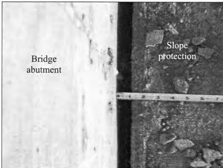
Figure 3.209 - Top View Showing Lateral Movement of the Abutment Away from the Bridge Embankment (Bridge No. 7777.0R065 - South End of NBL)
