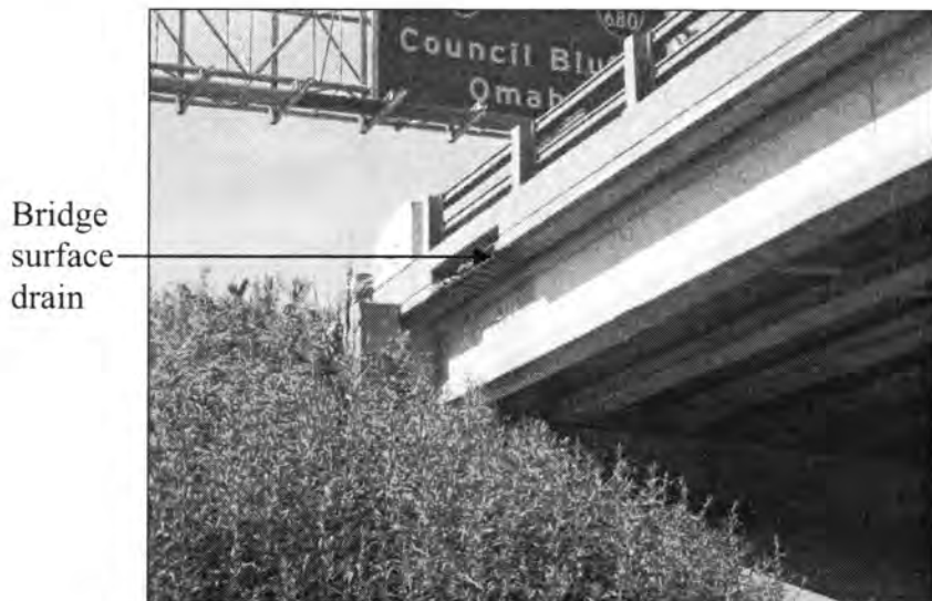
Figure 3.70 - Surface Drain of the Bridge Deck Allowing Water to fall on the Embankment (Bridge No. 78071.5R29)
