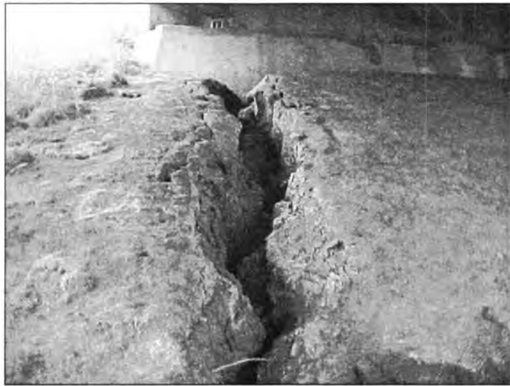
Figure 3.13 - Soil Erosion Under the Bridge (Bridge at U.S. 65 over Rail Road - North End of SBL)
