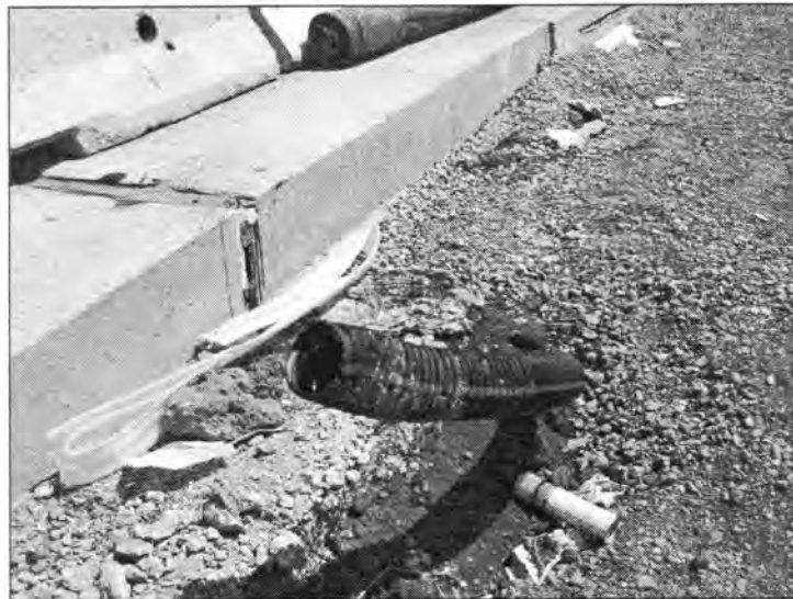
Figure 3.156 - End Drain Outlet Filled with Soil (Euclid Avenue Bridge)
