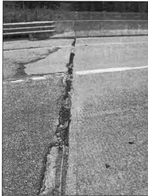
Figure 3.91 - Poorly Resurfaced Approach Slab (Bridge No. 9266.2R - West End of WBL)
