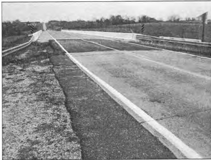
Figure 3.19 - Recently Placed Asphalt Overlay at the Bridge Approach (Bridge Carrying 72 nd St. over I-35 - East End)
