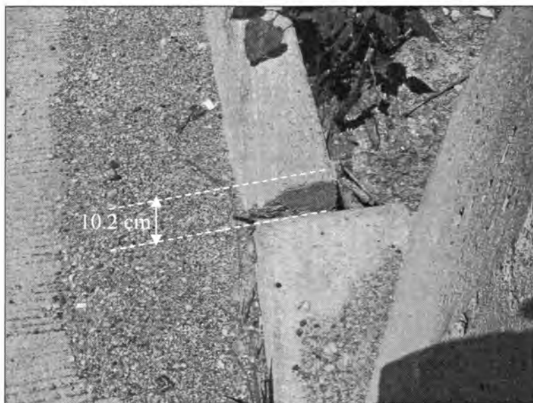
Figure 3.202 - Differential Settlement at the Bridge Approach (Bridge No. 7777.0R065 - North End of NBL)
