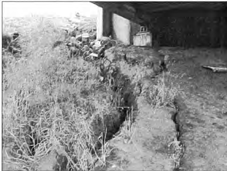
Figure 3.17 - Soil Erosion of the Bridge Embankment (Bridge No. 8556.8L030)
