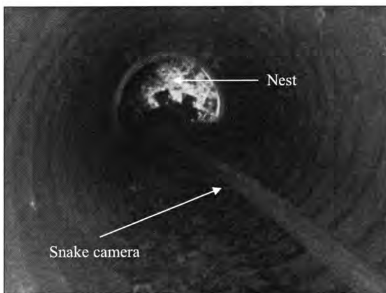
Figure 3.230 - Rodent Nest blocking the Subdrain at 1.5 m from the Outlet (Bridge No. 7779.0065)
