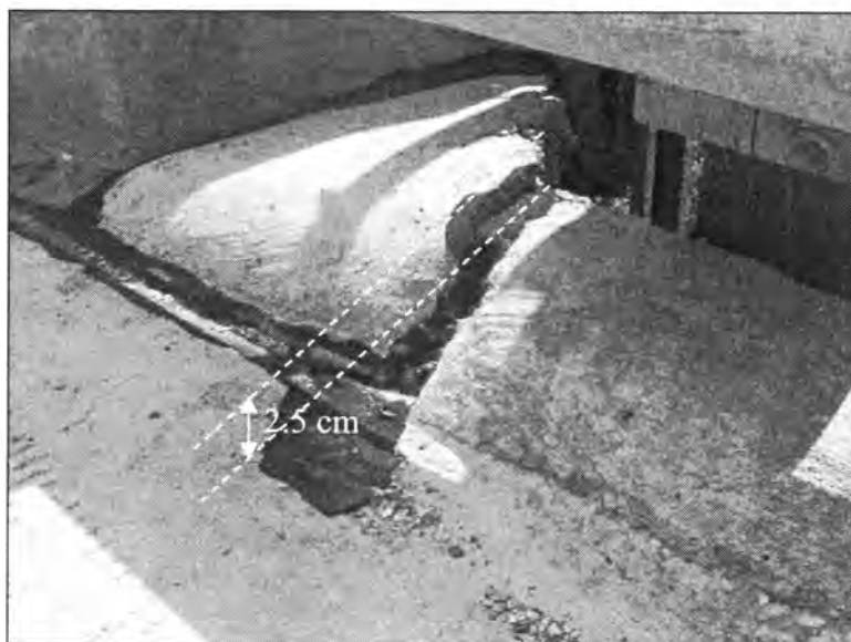
Figure 3.192 - Differential Settlement between the Bridge Deck and the Bridge Approach (Bridge No. 7773.0R065 - South End of SBL)
