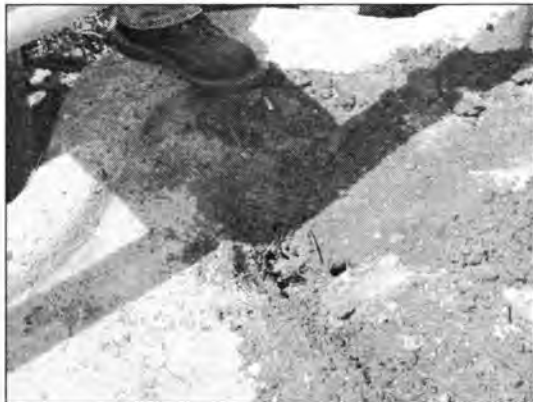
(a) Bridge End Drain Blocked by Debris
