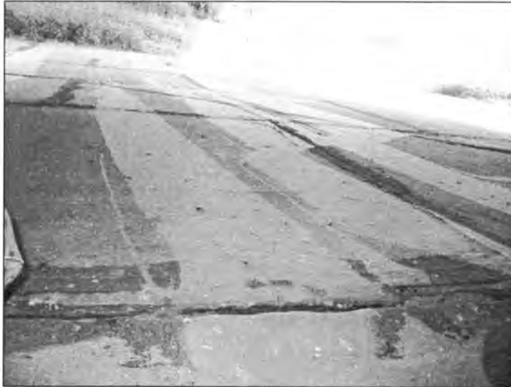
Figure 3.99 - Grout Seeping from under the Concrete Cover (Bridge No. 574.2S001)
