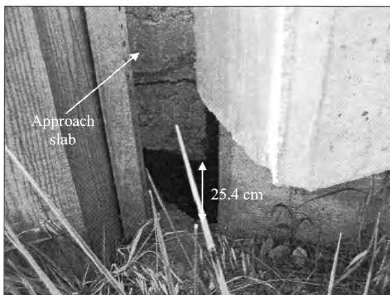
Figure 3.204 - A Void Developed under the Approach Slab (Bridge No. 7777.0R065 - South End of NBL)
