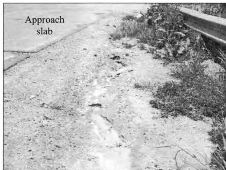
Figure 3.55 - Erosion Caused by Runoff Water at the Approach Slab Shoulder (Bridge No. 982.9)
