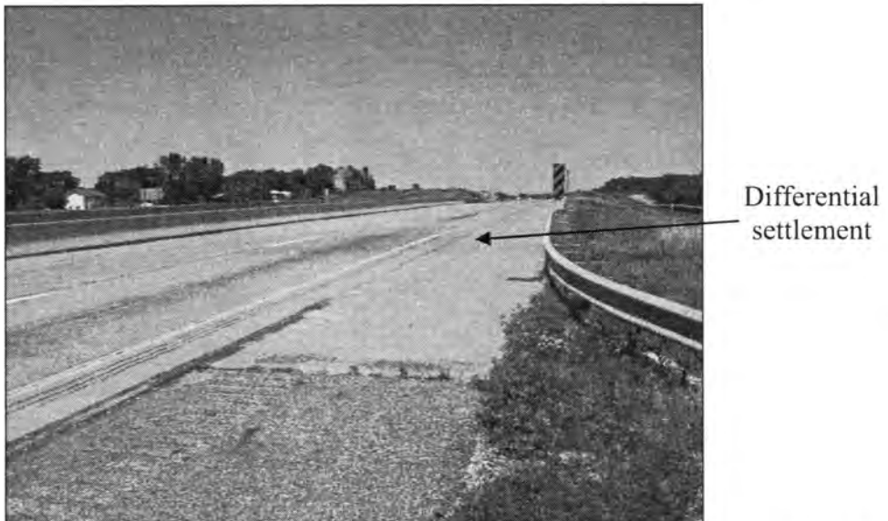
Figure 3. 221 - Differential Settlement of the Approach Slab (Bridge No. 7778.1065 - North End of SBL)
