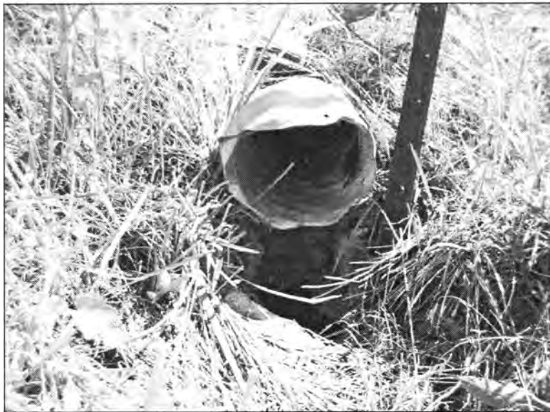
Figure 3.198 - Subdrain Prior to Insertion of Snake Camera (Bridge No. 7773.0R065 - North End of NBL)
