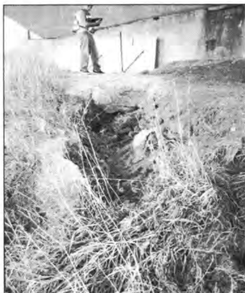
Figure 3.37 - Erosion of the Embankment Soil under the Bridge (Bridge No. 1270.2S014)
