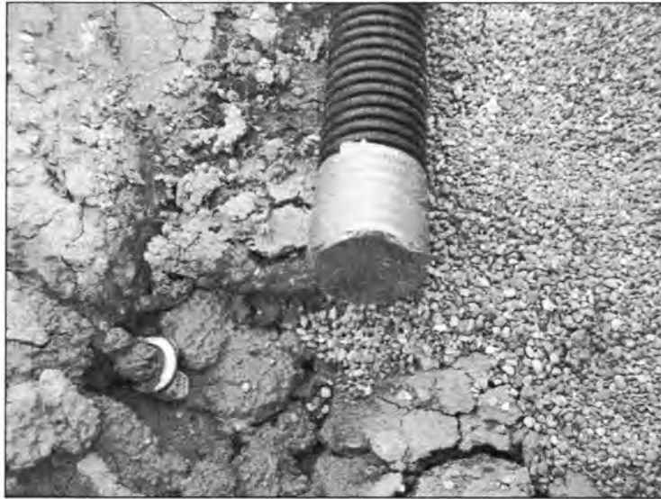
Figure 3.120 - Porous Fill Placed around the Subdrain (35 th Street over I-235)
