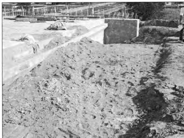
Figure 3.163 - Poorly Placed Granular Backfill (Bridge over Union Pacific Railroad)
