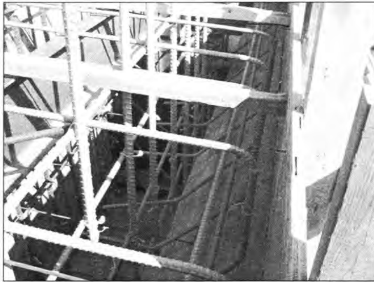
Figure 3.150 - Abutment and Paving Notch Rebars Tied with Reinforcement from the Backwall (East 12 th Street Bridge)
