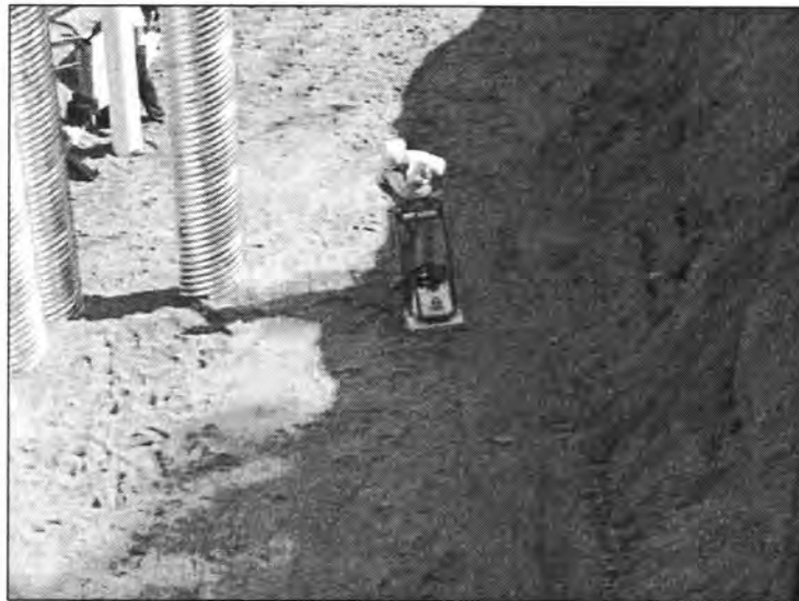
Figure 3.136 - Compaction of Retaining Wall Fill Material (Polk Blvd. Bridge - South End of SBL)
