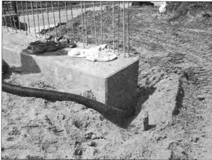
Figure 3.133 - No Porous Fill Surrounding the Subdrain (Polk Blvd. Bridge - North End NBL)
