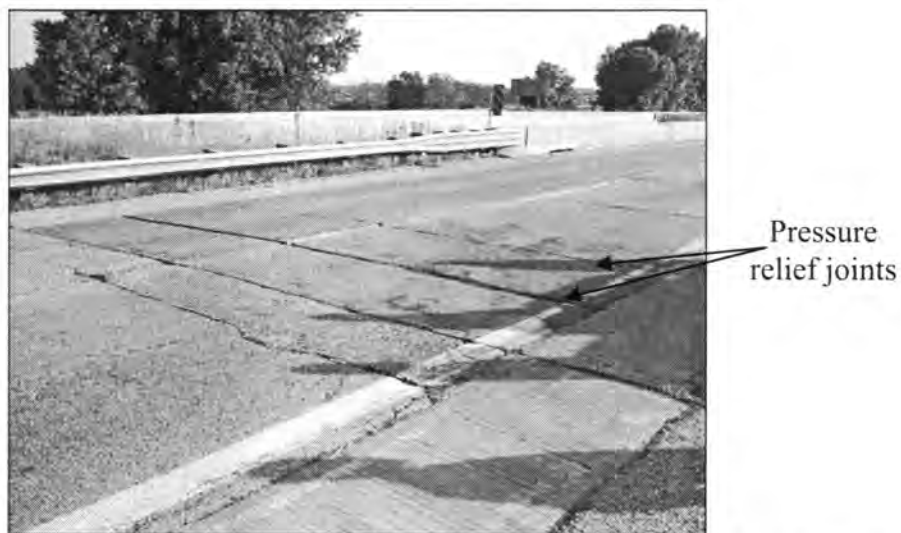
Figure 3.62 - Pressure Relief Joint Made by Cutting the Approach Slab (Bridge No. 786.8R080)
