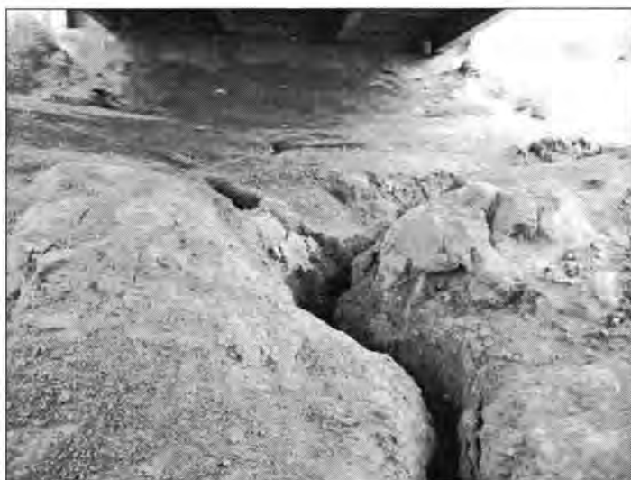
Figure 3. 59 - Soil Erosion of the Embankment under the Bridge (Bridge at U.S. 20 over West Fork Little Sioux River)
