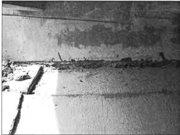
Figure 3. 52. Uneven Settlement of slope protection (Bridge No. 9702.9)
