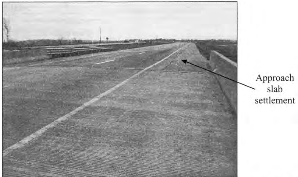
Figure 3.174 - Settlement of Approach Slab (Bridge No. 76.8065 - North End NBL)
