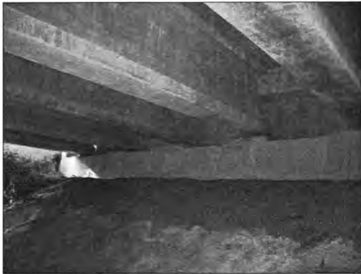
Figure 3.98 - Wet Loess Soil Observed at the Bridge Embankment (Bridge No. 574.2S001)
