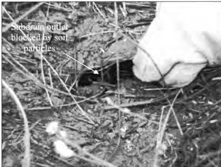
Figure 3.246 - Subdrain Outlet, Located at the Bottom of the Embankment, Blocked by Soil Particles (Bridge no. 7779.4065)
