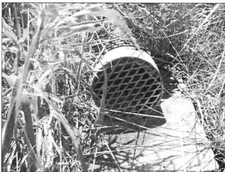
Figure 3.194 - End Drain in a Satisfactory Condition (Bridge No. 7773.0R065 - South End of SBL)
