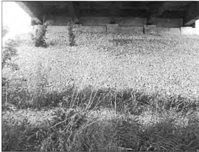
Figure 3.200 - Aggregate Slope Protection at the Bridge Embankment (Bridge No. 7774.0L065 - North End of NBL)
