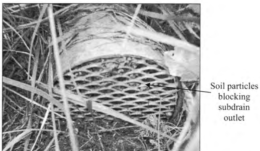
Figure 3.94 - Subdrain Outlet Blocked with Soil Particles (Bridge No. 9266.2R - West End of WBL)
