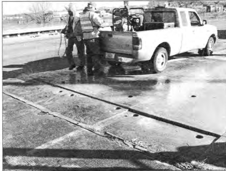
Figure 3.30 - Section of the Approach Slab Cut and Ready to be Removed (Bridge Carrying 160 over I-35)
