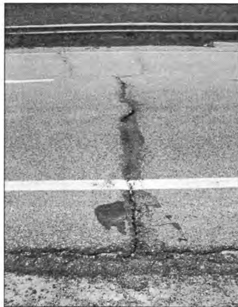
Figure 3.92 - Transverse Cracking of the Asphalt Overlay (Bridge No. 9266.2R - West End of WBL)
