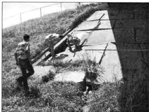
(a) Damaged Slope Protection
