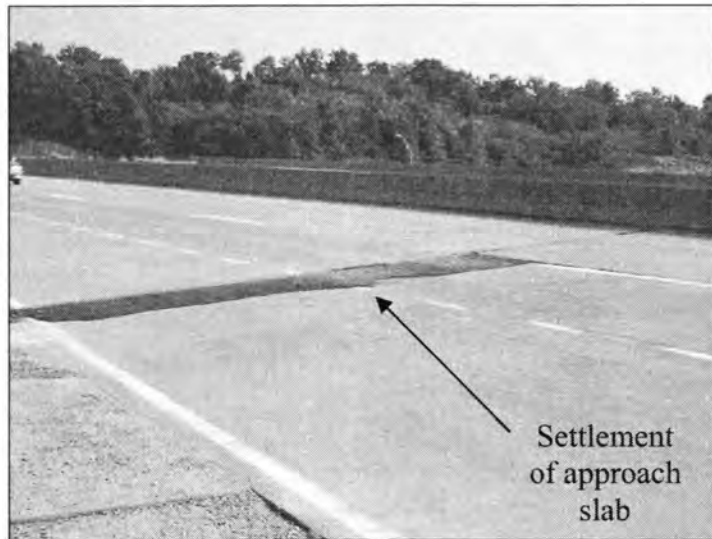
Figure 3.102 - Differential Settlement at the Approach Slab (Bridge No. 574.2S001)
