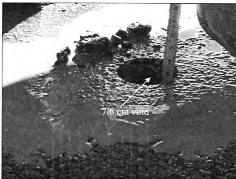
Figure 3.223 - A 7.6 cm Void under the Approach Slab Estimated by Measuring the Distance the Core Dropped (Bridge No. 7778.1065 - North End of SBL, Edge Line)
