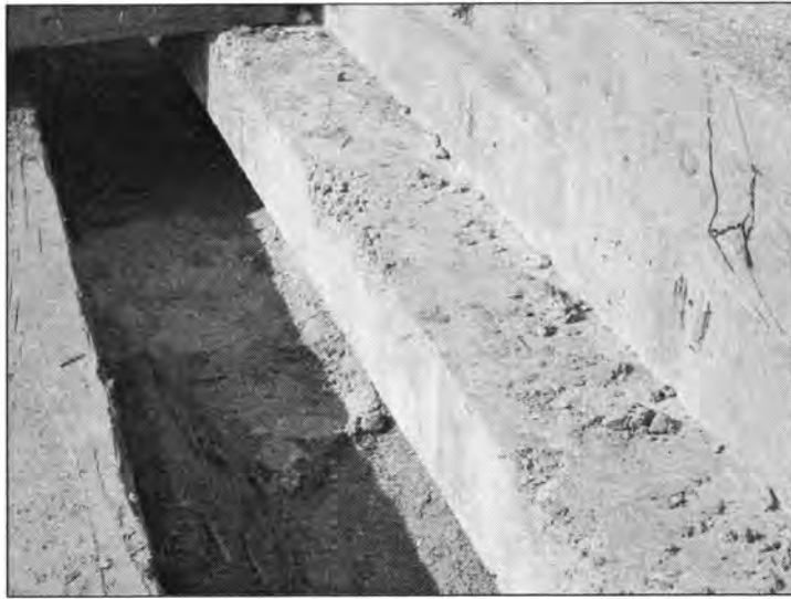
Figure 3.165 - Poor Construction of Paving Notch (Bridge over Union Pacific Railroad)
