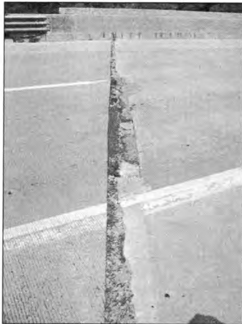
Figure 3.108 - Concrete Spalling and Cracking at the Expansion Joint (Bridge No. 5200.5R380)
