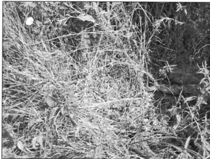
Figure 3.66 - Drainage Outlet Could Not be Located (Bridge No. 788.5R080)
