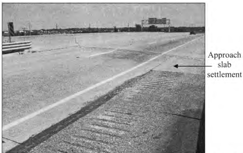
Figure 3.258 - Settlement of the Bridge Approach (Bridge No. 7782.8L065 - North End of SBL)
