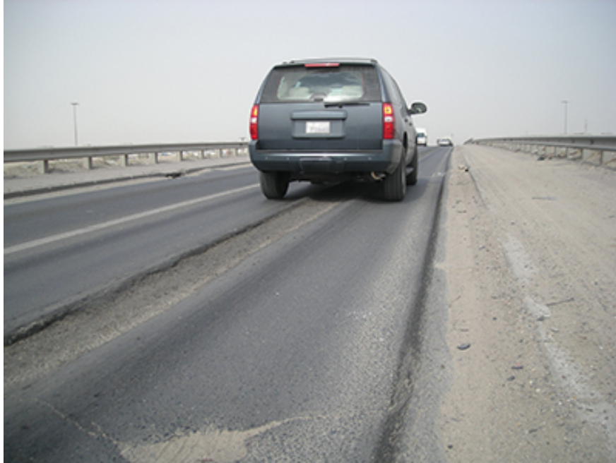
Figure 1.1: Rutting happening in an asphalt pavement under the wheelpath.
