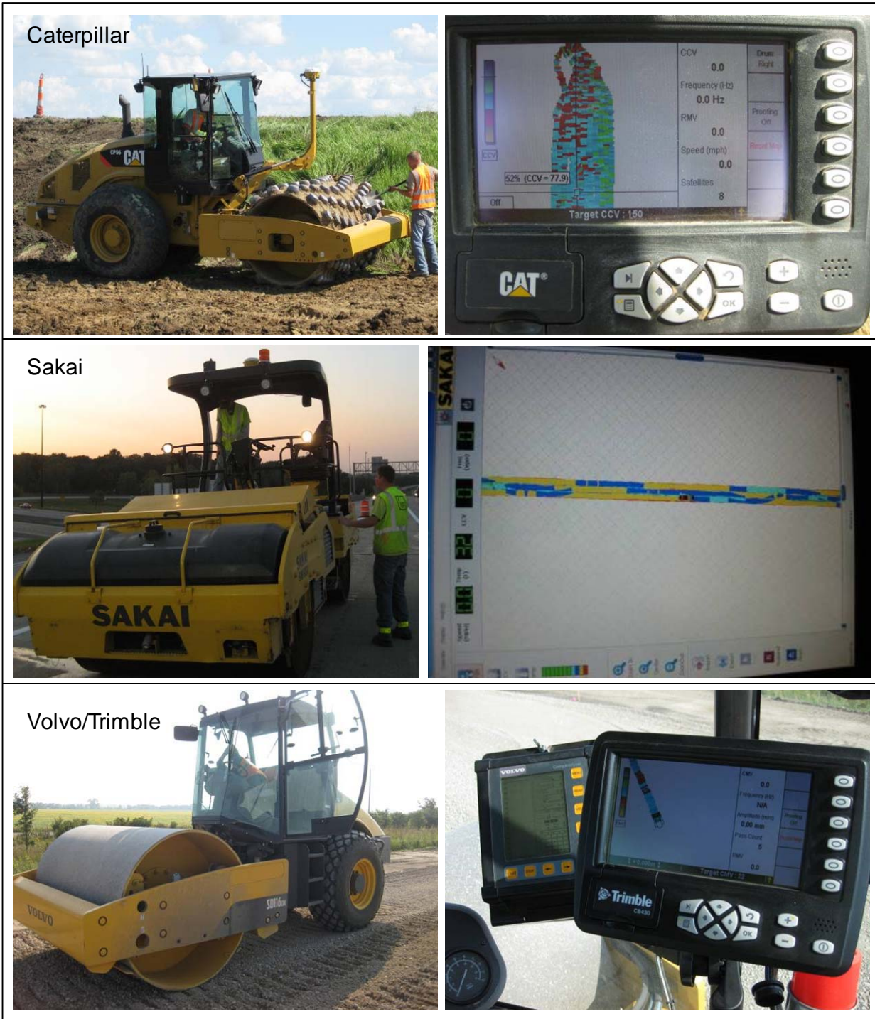
Figure 1. Caterpillar CP56 (top) padfoot roller with onboard AccuGrade display unit used on US30 project, Sakai SW880 (middle) dual smooth drum roller with onboard Aithon MT display unit used on US218 project, and Volvo SD116DX (bottom) roller with onboard Trimble CB430 display unit used on I29 project
