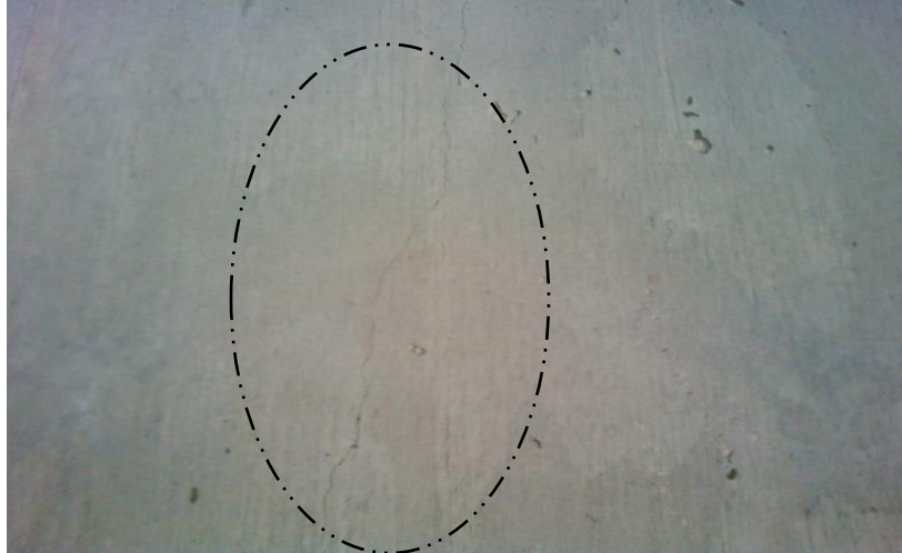
Figure 4.1. North abutment hairline crack
