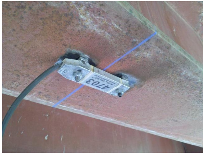
Figure 5.29. Mounted strain transducer
