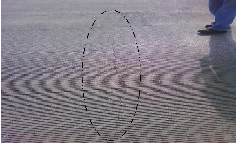
Figure 4.4. Deck transverse cracking
