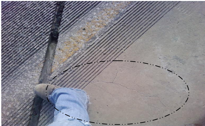
Figure 4.3. Off-ramp slab cracking
