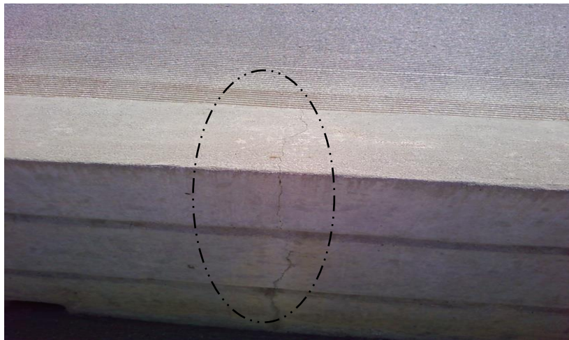
Figure 4.5. Guardrail transverse cracking
