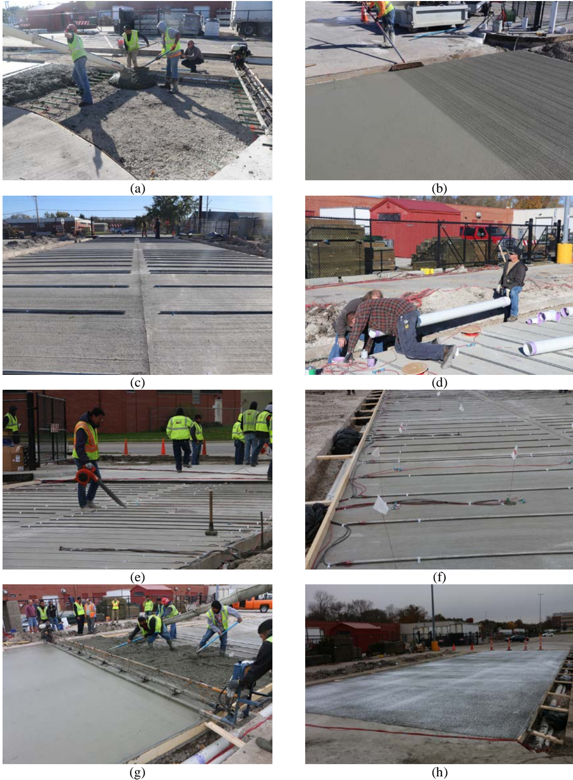
Figure 4 ECON HPS construction steps: (a) C-3WR-C20 PCC placement, (b) PCC layer screeding, (c) electrode installation, (d) PVC conduit placement, (e) surface cleaning, (f) ECON layer before placement, (g) ECON placement and compaction with vibrating screed, and (h) curing compound spraying.
