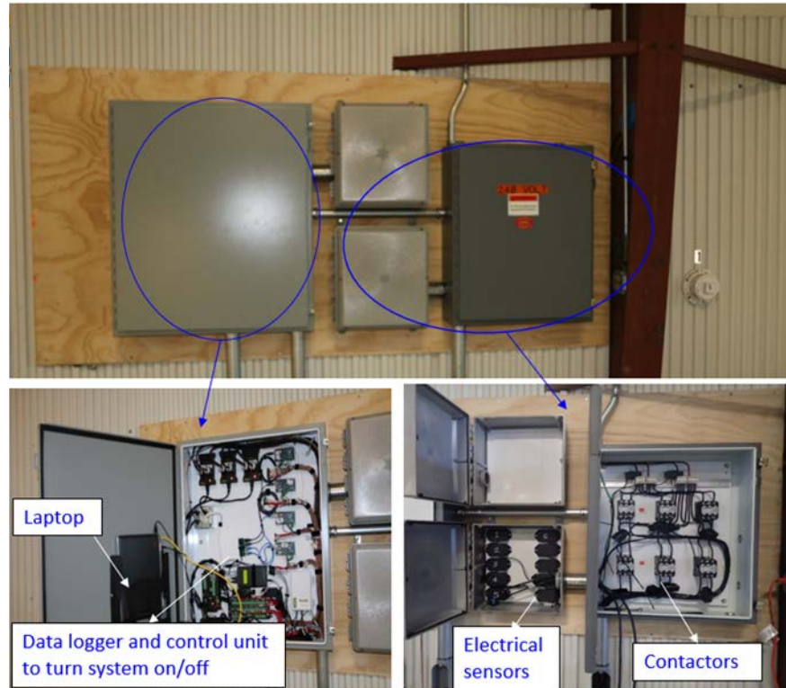
Figure 5-5 Power supply panel integrated with remote monitoring control system
