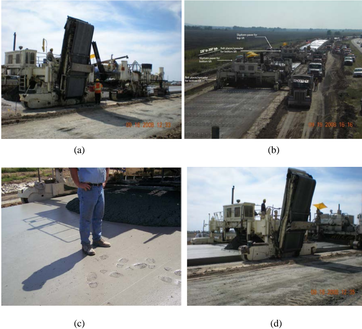
Figure 2-7 Two-lift construction of concrete pavement in progress: (a) two-lift paving equipment train, (b) bottom lift belt placer/spreader and paver, (c) demonstration of the concrete stiffness of the bottom lift, and (d) top lift belt placer/spreader and paver (Hu et al. 2014 and Gerhardt 2013)
