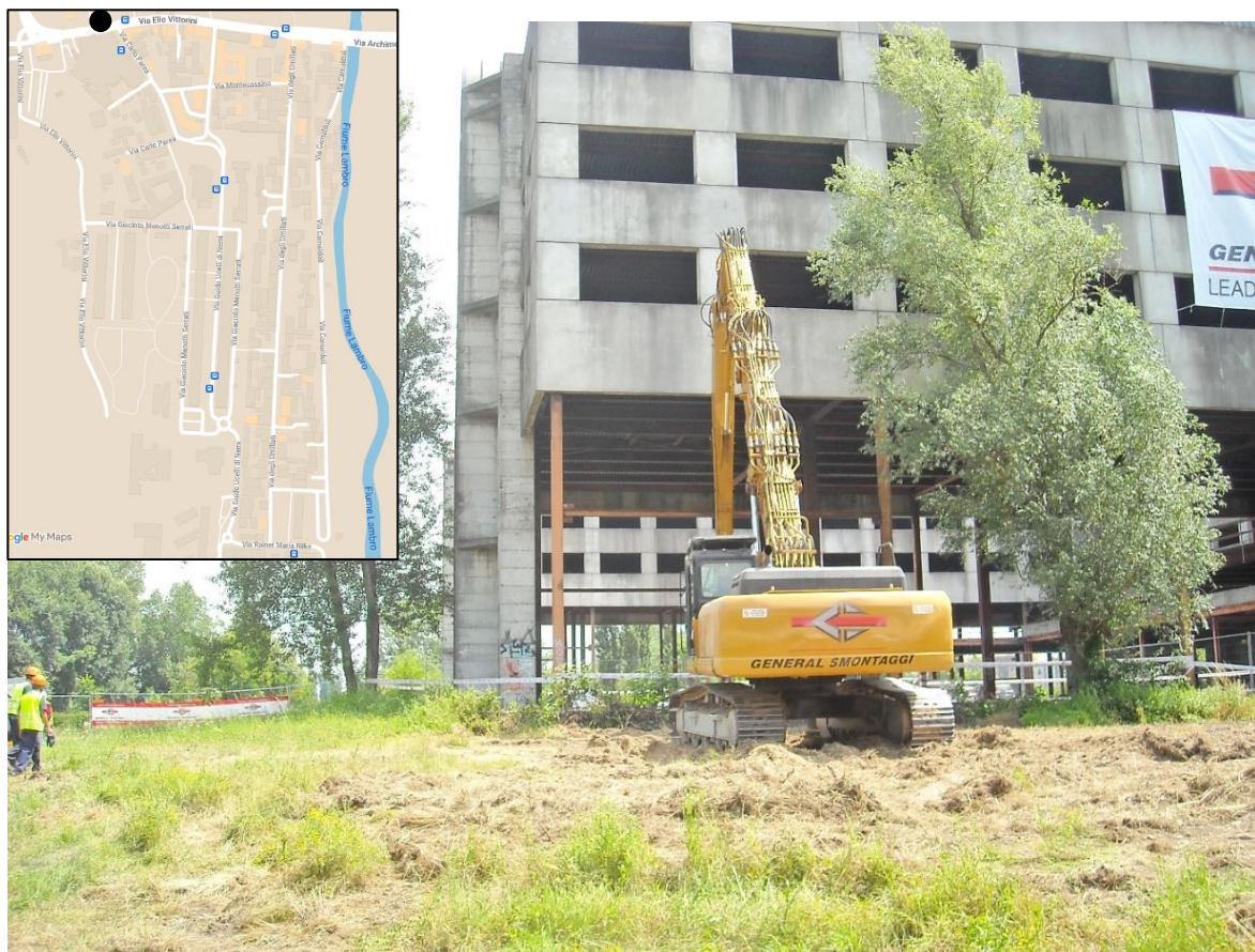
Photo 14. "Abattimento ex Albergo Mondiali - Demolition of former World Cup Hotel" (Source: Carlo, current long-term resident, over 60).
