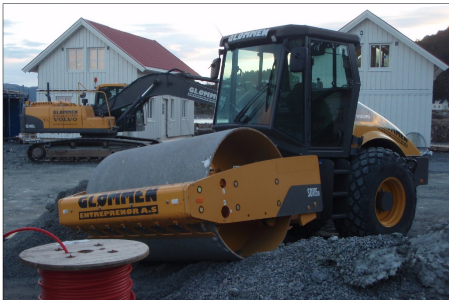
Figure 6.5. Vibratory roller Volvo SD115D used at Statland when compacting a road fill (photo NVE).
