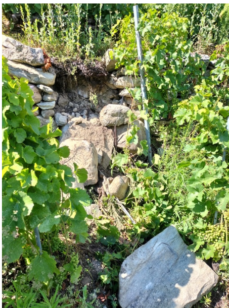
Figure 32. Dry-stone wall crumbled apart (source, P5).
