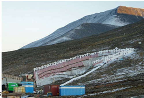
Figure 9. For protection of the entrance to the Svalbard Seed Vault, a 20 m high frozen wall is created to stabilize the permafrost [19]. (Photo: Thomas Nilsen, Barents Observer)
