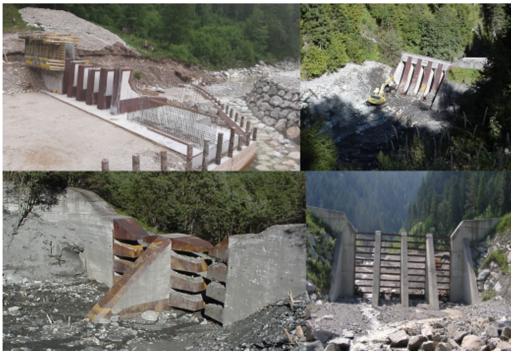
Fig. 1 Active debris-flow specific mitigation measurements in torrents. Above from left to right: Rindbach (Upper Austria-AT); Luggauerbach (Salzburg-AT). Below from left to right: Luggauerbach (Salzburg-AT); Naisbach (South Tyrol-IT)
