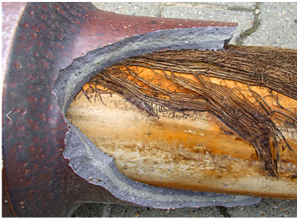
Fig. 7. Root ingrowth between liner and host pipe.
