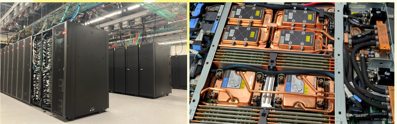
Left: A look inside the Data Centre that houses BlueBEAR. Right: A closer look: internal workings of a HPC node
