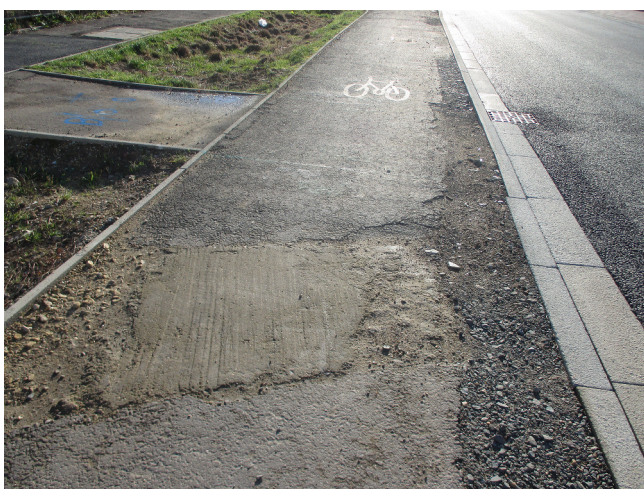
Fig. 4. Unfinished terrains, photographed by Tom “There’s a lot of holes there as well on the path which is quite irritating because like it’s gravelly. One of my friends fell here actually like because of a stone, like the tyre slipped.” (Tom, age 12, Northstowe).
