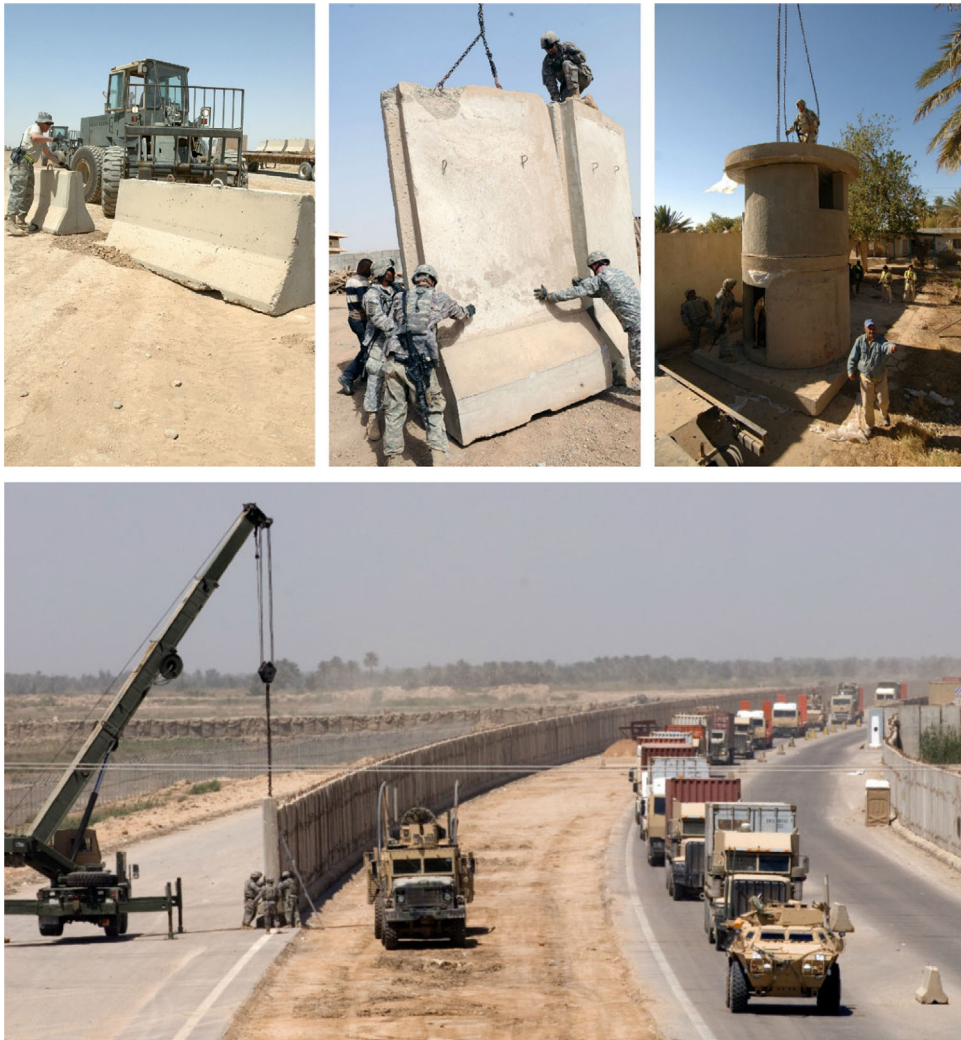
Figure 1: Top—Images of emplacing [i] Jersey walls (far left), [ii] Alaska blast walls (centre), and [iii] guard towers used at checkpoints (far right) in Iraq 2008. Image credit: Senior Airman Eunique Stevens, US Air Force; Staff Sgt. James Selesnick, US Army (source: Spencer 2016). Bottom—the US military’s tactic of lining every major road with T-walls. Image credit: Spc. Kiyoshi Freeman, US Army (source: Spencer 2016).
