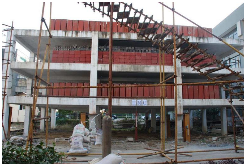
Figure 2. 17 Half-scale reinforced concrete frame retrofitted with carbon-reinforced strip cables progressive collapse column removal test (Liu et al., 2017)
