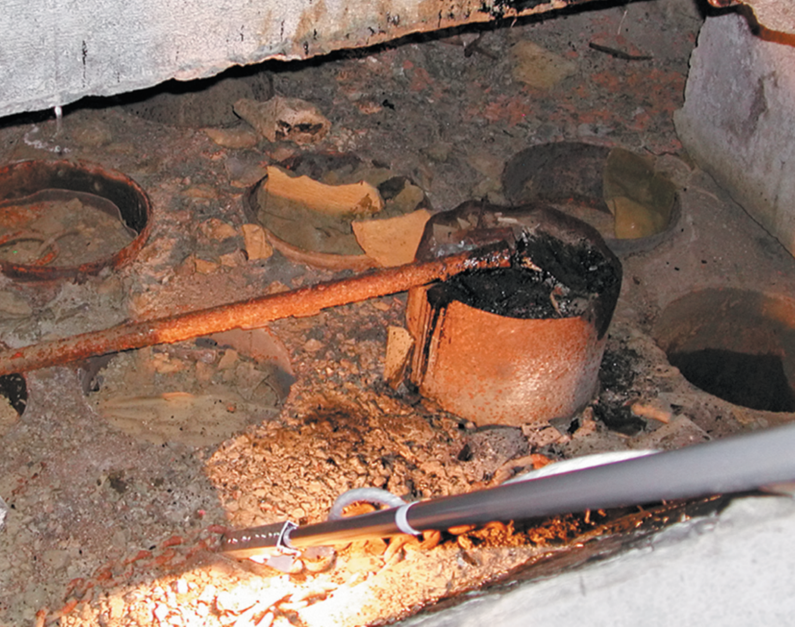
Cells of a dry spent fuel storage facility in Andreeva Bay, 2001. Photo from the Bellona archive.
