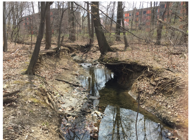
FIGURE 8 Channel enlargement (location of tree roots indicate original location of channel bank) caused by urban runoff in an urban stream in Baltimore, Maryland [Photo Source: Allen Gellis (USGS) as appear in Figure 2B of Gellis et al. (2020)].
