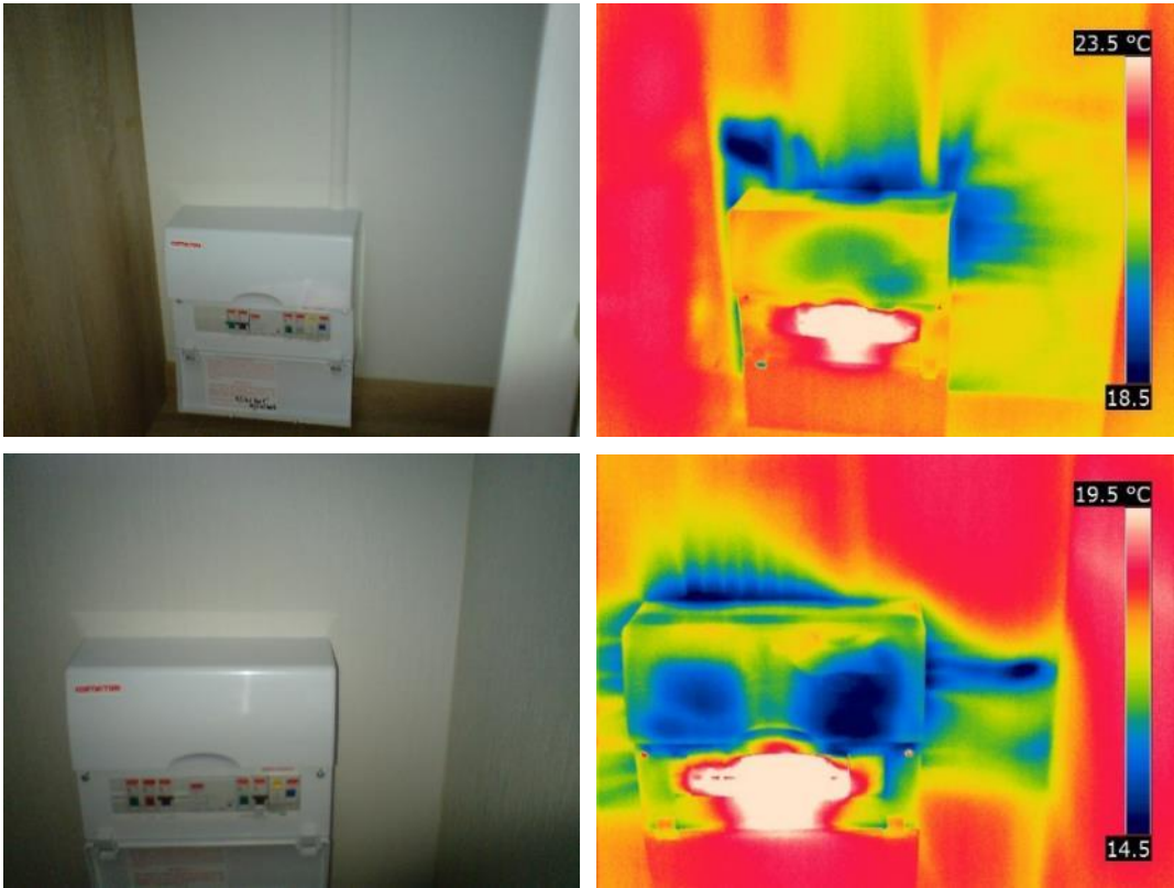
Figure 12 Air leakage around the consumer unit.
