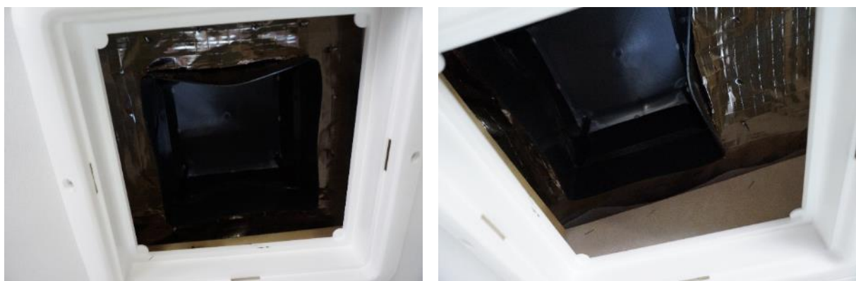
Figure 51 Lack of insulation around ceiling extract vent in kitchen area of caravan B.
