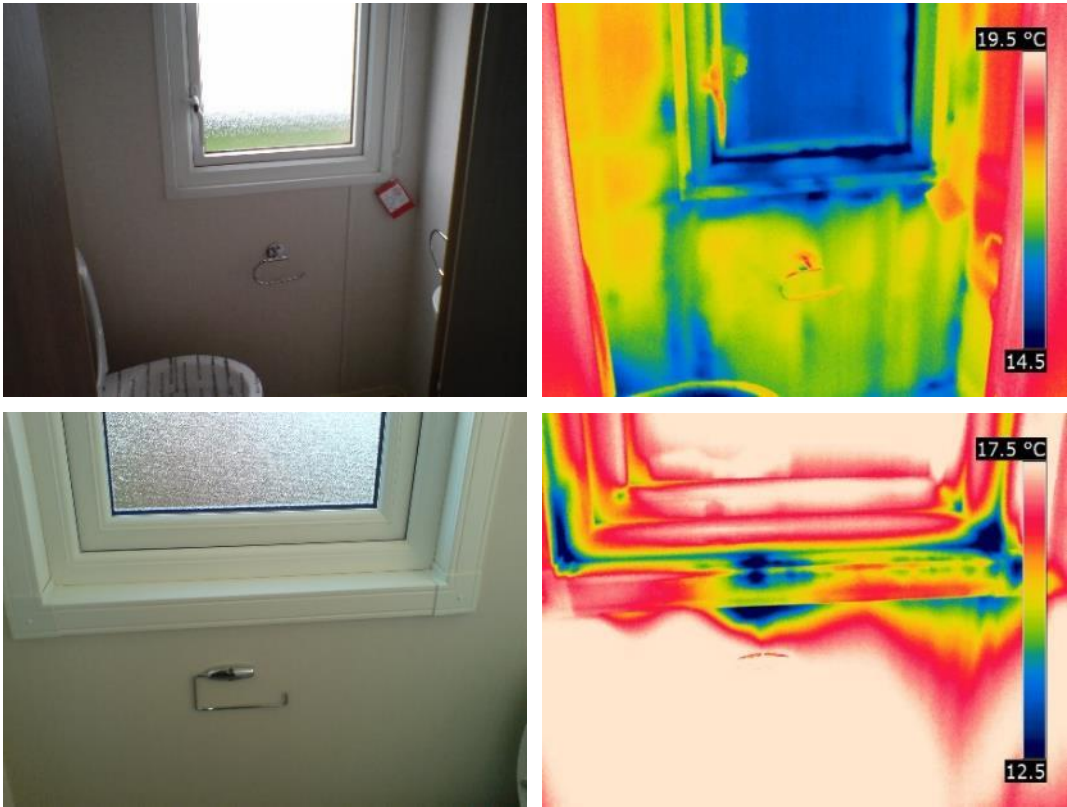
Figure 22 Air leakage around the window frames.
