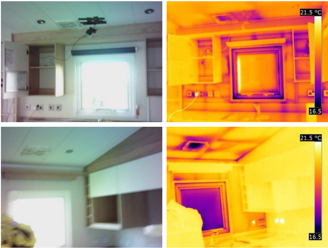
Figure 33 Thermal bridging around the ceiling mounted extract fan in the kitchen/living area.
