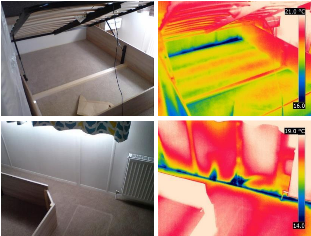
Figure 24 A leakage at the external wall/floor junction in the master bedroom of caravan A (top) and caravan E (bottom).
