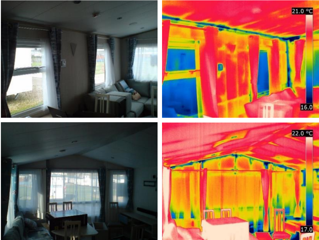
Figure 20 Air leakage at the external wall/ceiling junction (top and bottom) and at external wall corners (top).
