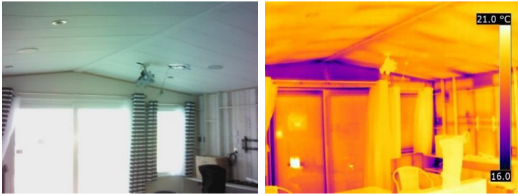
Figure 41 Thermal bridge at the sloping section of the kitchen/living area end wall in caravan A.
