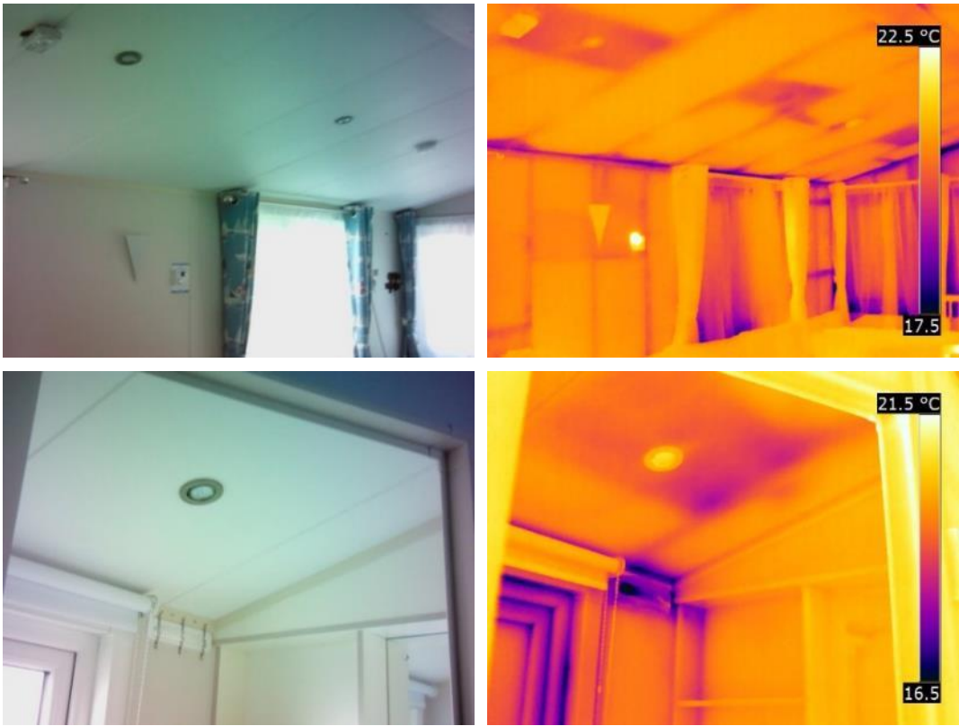
Figure 35 Thermal bridging around spotlights.
