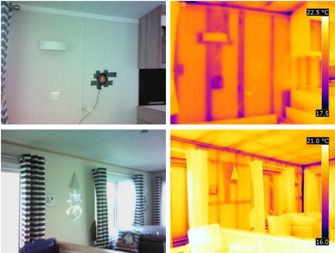
Figure 36 Thermal bridging around wall and light switches, particularly where there are cable runs.
