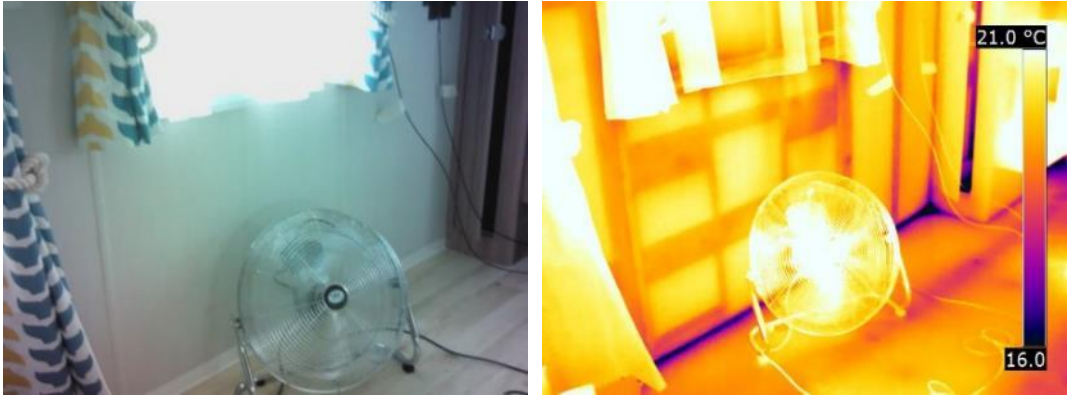
Figure 39 Thermal bridging below the kitchen/living area window in caravan E.
