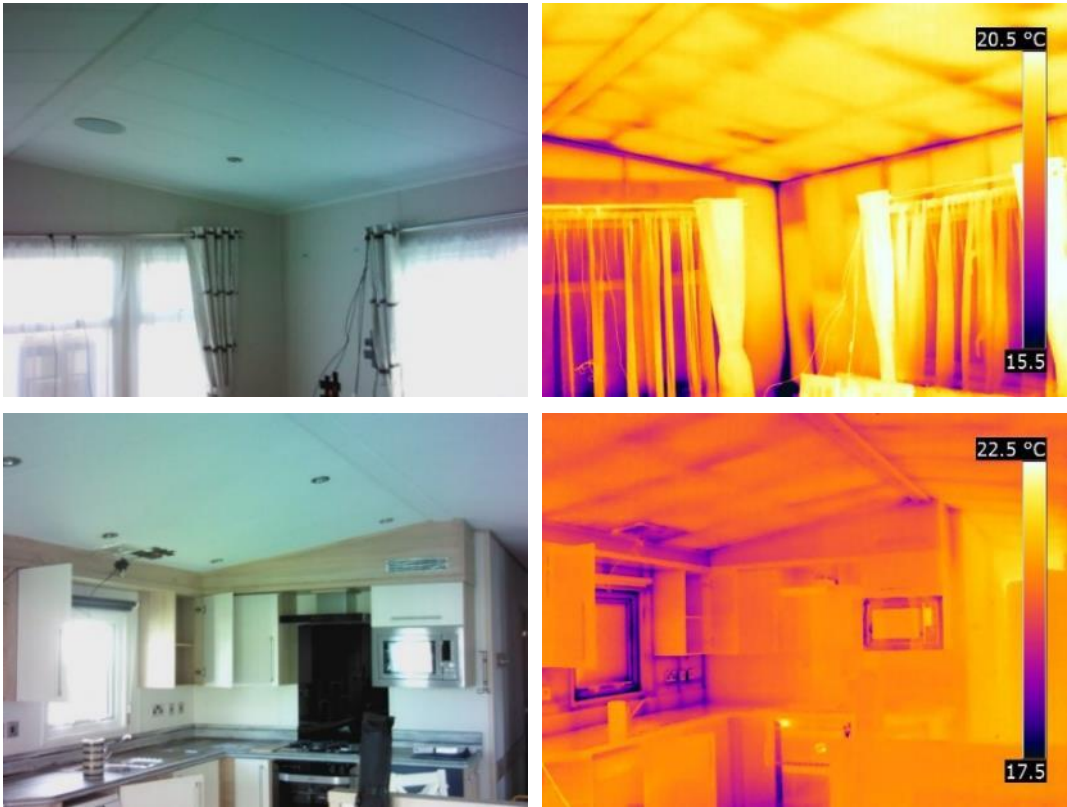
Figure 32 Thermal bridging at the roof joists and noggins.
