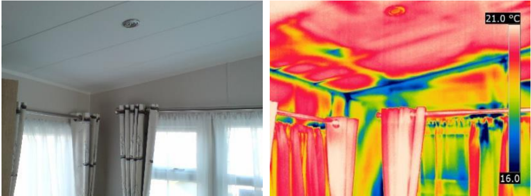
Figure 21 Air leakage at the external wall/ceiling junction in caravan D.
