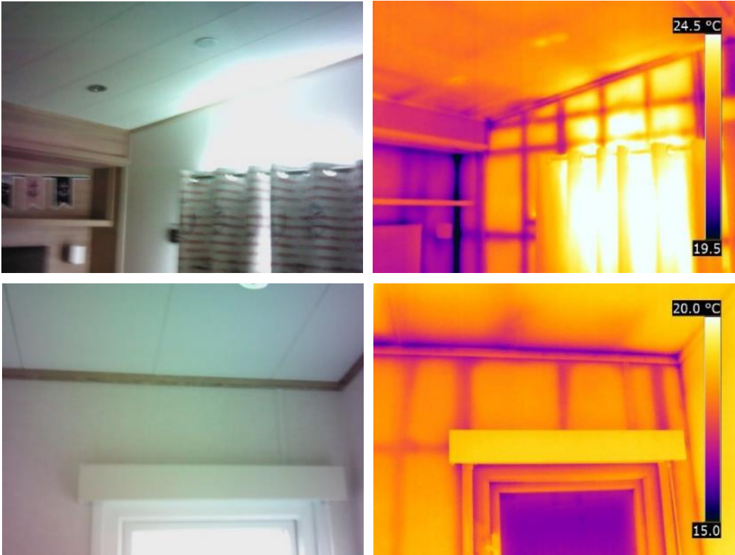
Figure 30 Thermal bridging at the vertical and horizontal studs in the external walls.
