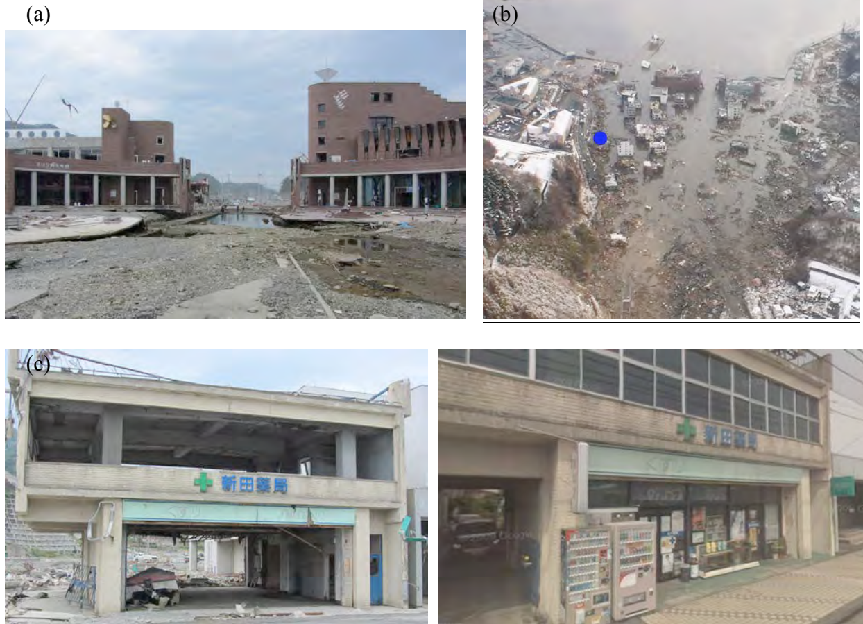
Figure 3. Tsunami destruction pattern in Onagawa ( 38^{\circ}26.5'N 141^{\circ}26.5'E ). (a) A pair of sturdy large buildings at the waterfront acted like barriers for some of the weaker buildings behind. (b) An areal view (the photo was enhanced from the original taken by Satake). The waterfront buildings can be identified in the photo. The gap between the buildings created a jet flow that completely destroyed the narrow strip of the jet trajectory, and caused a deep scour hole in-between. The blue circle shows the location of the toppled building shown in Fig. 2d, approximately 200 m from the waterfront. (c) The RC building severely damaged but standing. The walls on the ground floor were punched away by tsunami. The right panel shows the conditions prior to the 2011 tsunami, taken from the GoogleMaps/StreetView.
