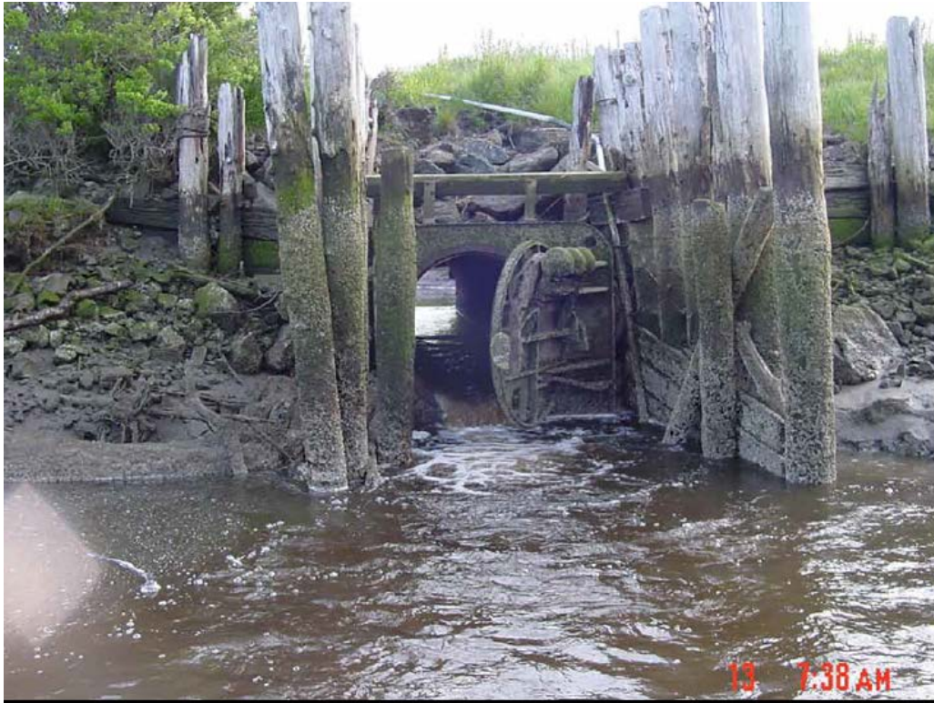
Figure 35. Fahys tide gate during mid-ebb tide in late spring. Note the elevation drop from the pipe to the pool level downstream.
