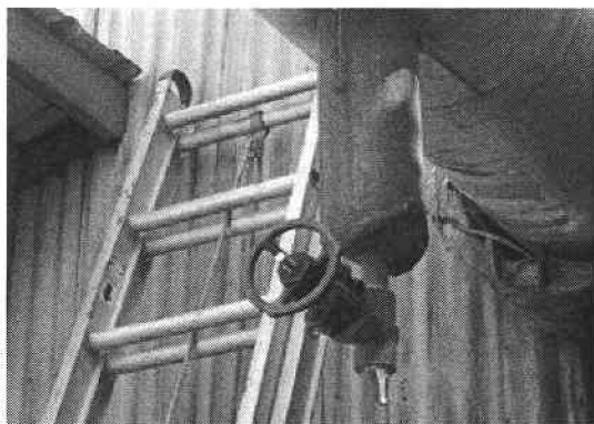
Mud legs & condensate lines.
