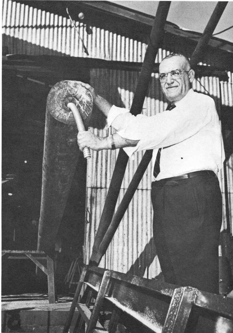
Milton H. Mater of Mater Engineering, Corvallis, Oregon, has solved the scenic pollution problem of what to do with utility wires while still utilizing wood poles. His firm developed a machine that bores 2 1/2 inch diameter holes lengthwise through poles 40 feet long. The wires are buried underground and concealed inside the poles through a conduit pipe. (Photo by Mater Engineering)
