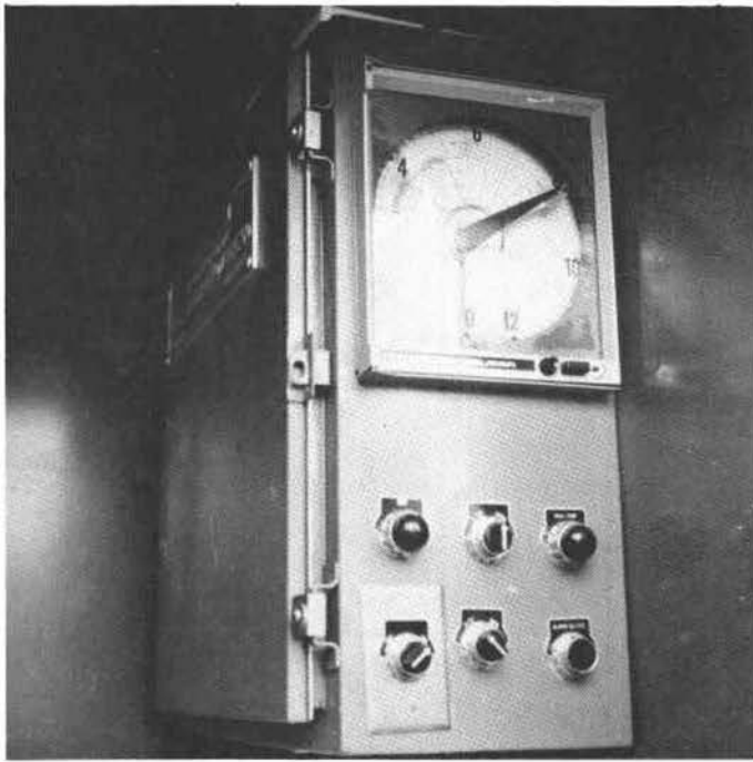
Figure 15. Temperature recorder-controller on a wigwam burner at Memphis, Tennessee.
