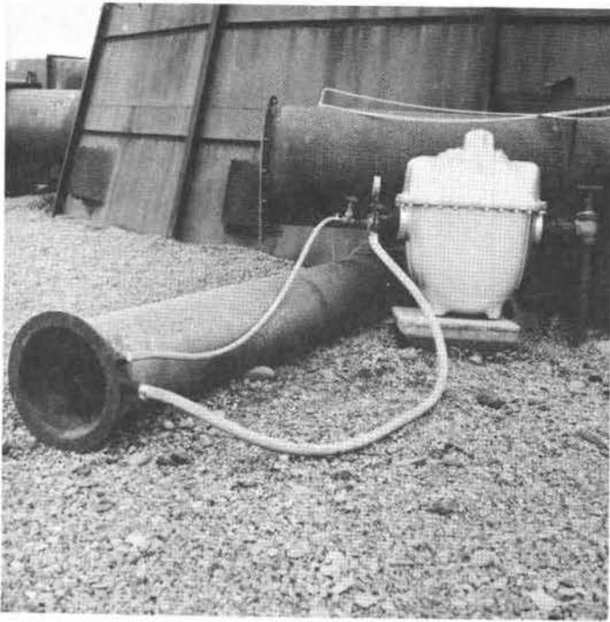
Figure 24. An auxiliary natural-gas burner duct (foreground) on the test burner.
