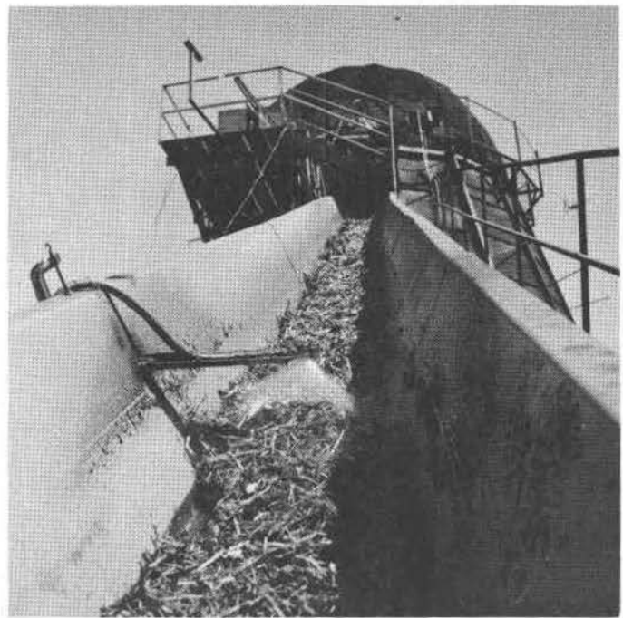
Figure 31. Water added to bark fuel going into the test burner.
