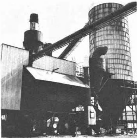
Figure 18. Automatically fired steam plant at a lumber mill in Grant's Pass, Oregon, that uses sawdust to produce steam for dry kilns.
