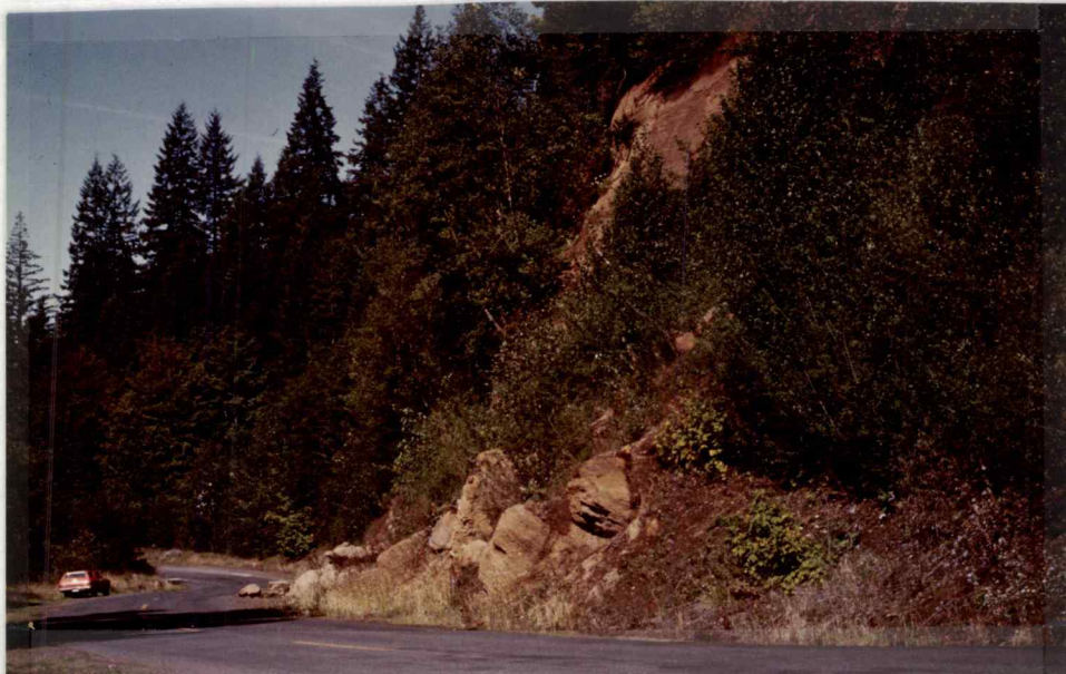
Figure 28. Rockfall-rockslide, developed in bedded sandstone of the Troutdale Fm., poses road maintenance problems (between the communities of Bull Run and Aims, west of the study area).
