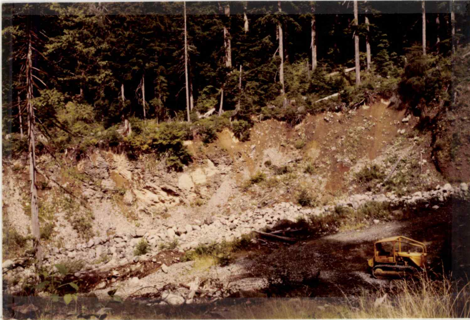
Figure 40. Streamside debris avalanche associated with North Fork debris torrent of January, 1972 (mass movement no. 6). Quaternary landslide debris is exposed in the failure surface. Rip rap has been placed along the toe to retard further stream undercutting.
